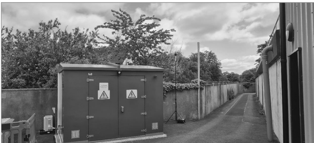
Location N6 -NSL
