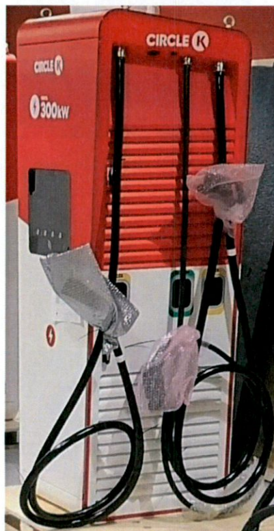
Figure 10: Typical Circle K Branded High Charging Unit
