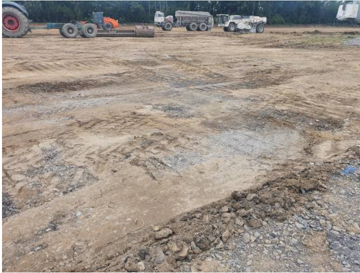
Plate 9 East side of the site showing the hardcore that may relate to the N82
