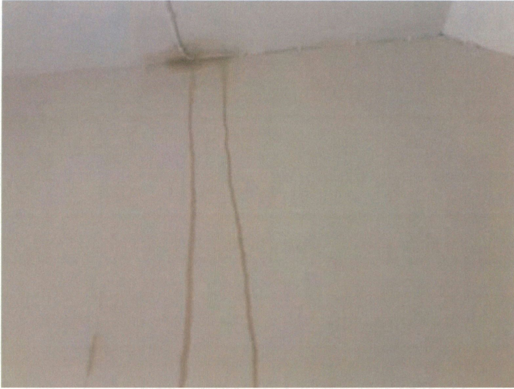
Photo 09 – Water ingress at chimney
