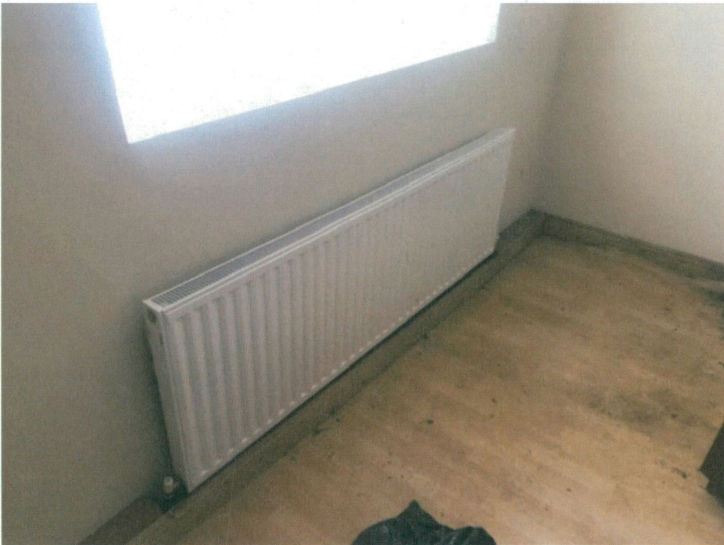
Photo 10 – Central heating in the second bedroom
