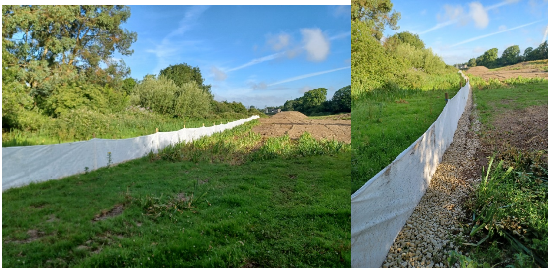
Figure 6.2: Silt fencing in situ River Camac (erected in place as part of the conditions of grant for both sites (Coffeys 13 th July 2022).
