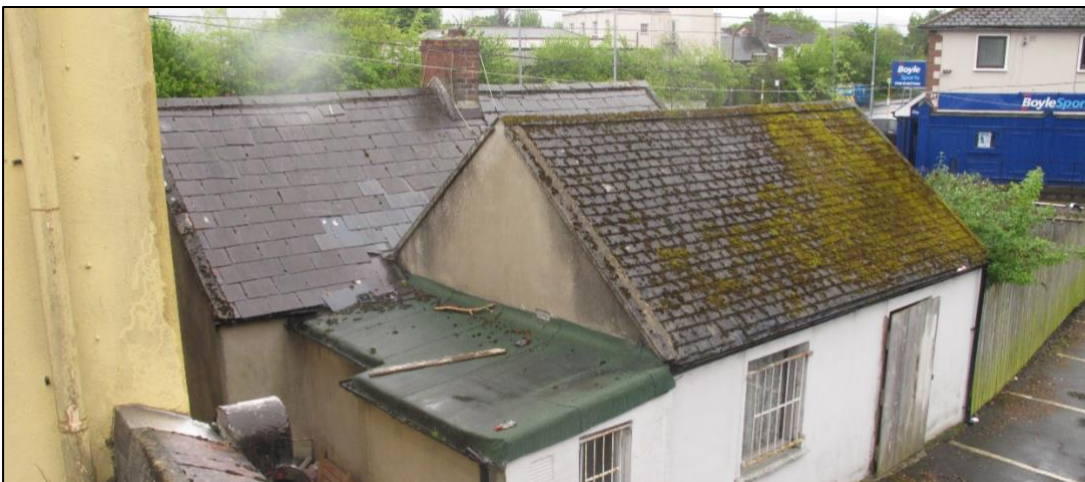
Plate 7. Cottage showing roof with valley between two attic spaces. Rear attic (right) is tiled. Front attic (left) is inaccessible and has several slates dislodged allowing possible entry of bats
