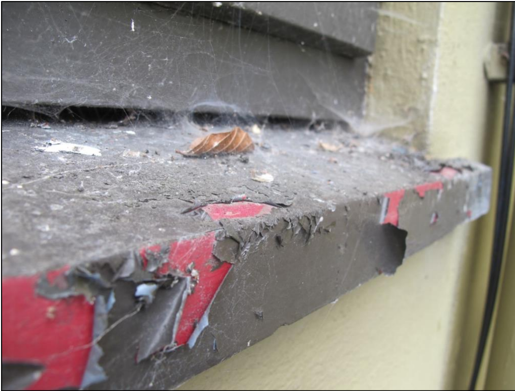
Plate 9. Exterior wall and windowsills were examined for bat droppings.
