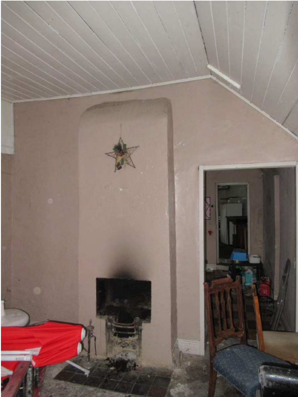
Plate No. 11. General internal view showing the chimney breast in the east room in the cottage. Note the timber-sheeted ceiling, with the collar ties raised above the wall heads.
