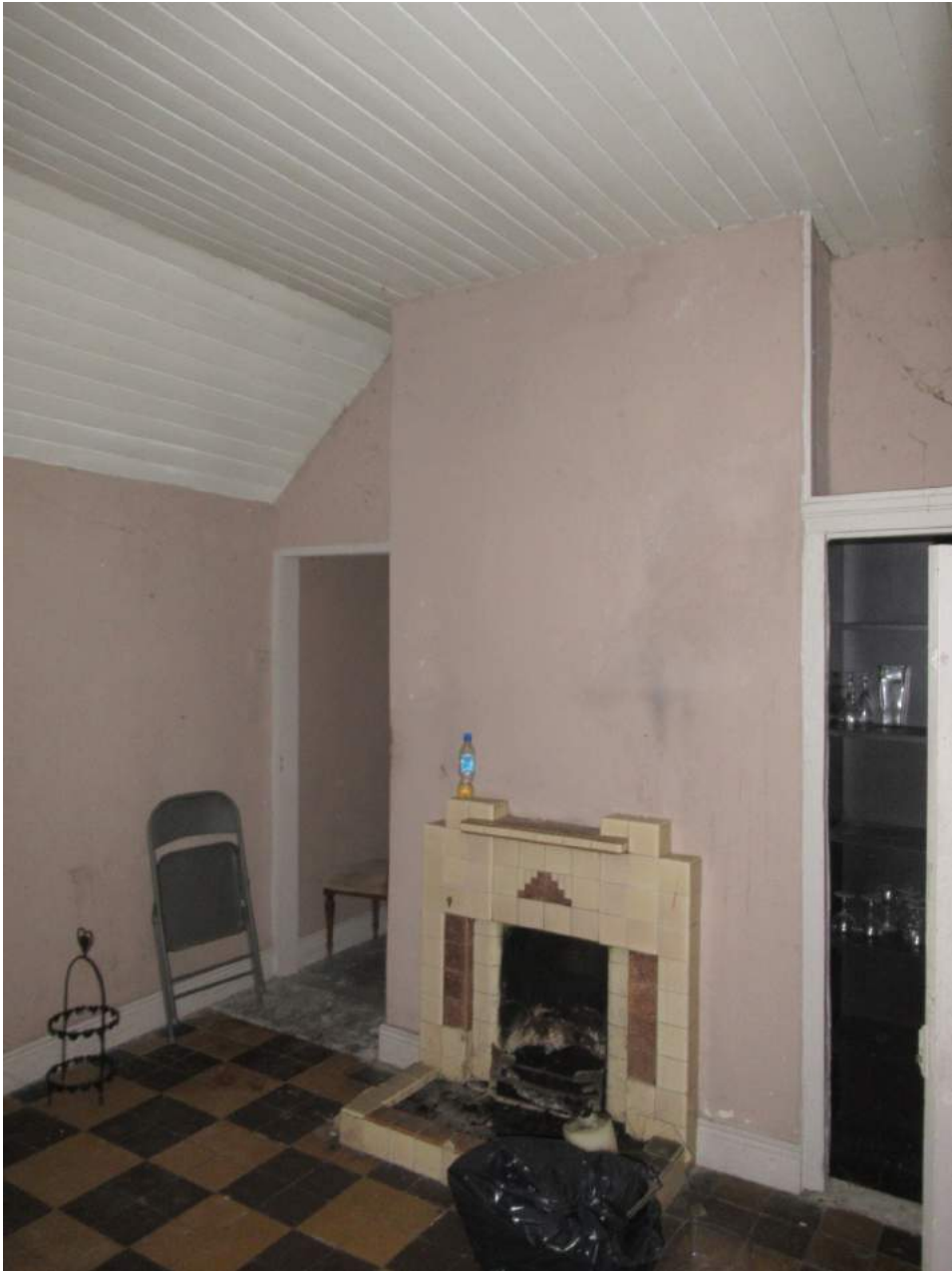
Plate No. 12. General internal view showing the fireplace in the west room in the cottage.
