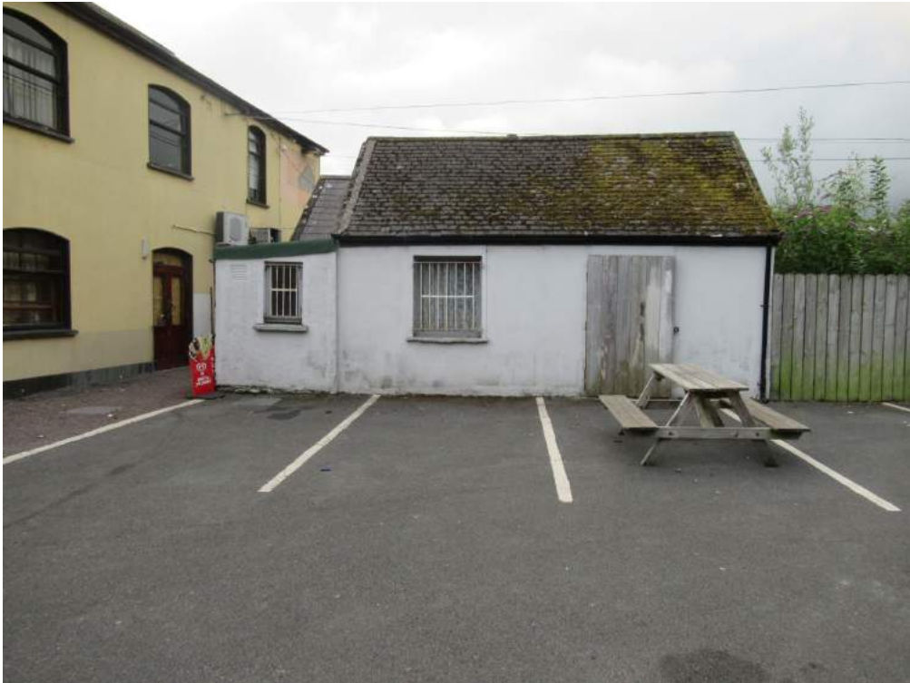
Plate No. 8. General view looking south showing the rear extension to the cottage.
