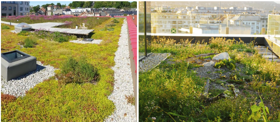
Figure 52. Biodiverse green-blue roofs. All roof penetrations such as rooflights or AOVs, as well as roof perimeters, should have a 300-500mm wide gravel strip to act as a firebreak
