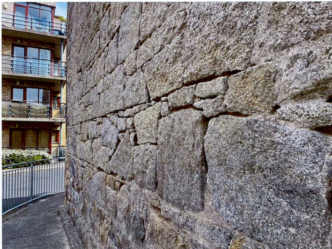
Photo 8: Detail of eroded joints to stonework to north gable
