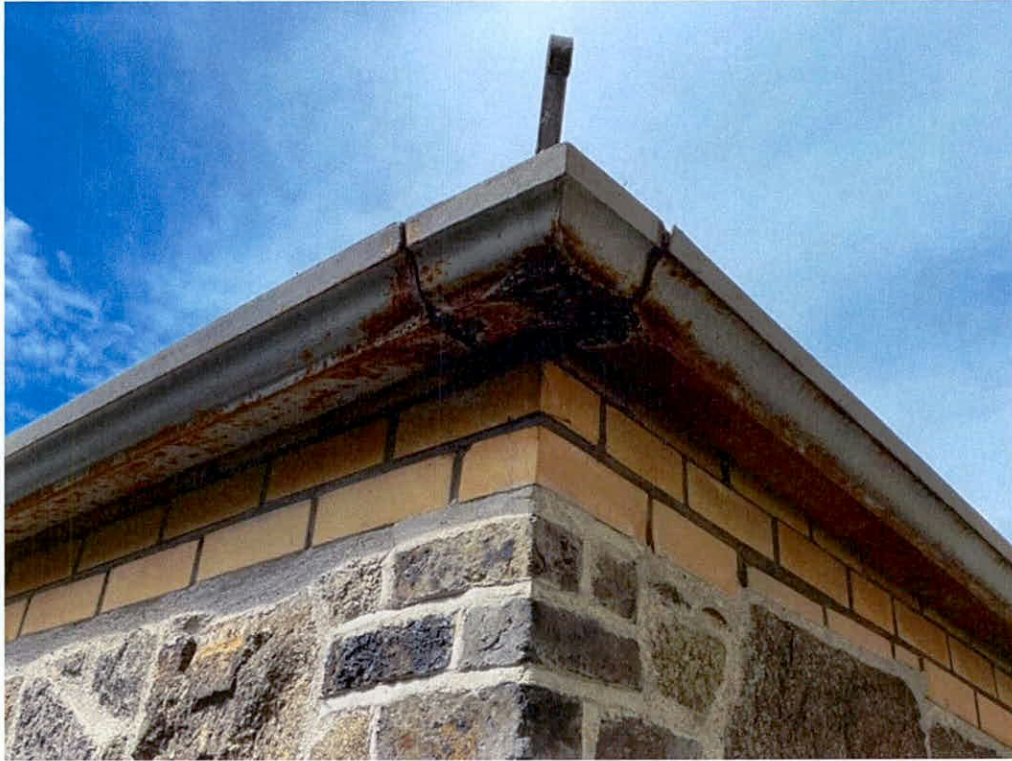
Photo 17: Detail of condition of cast iron guttering
