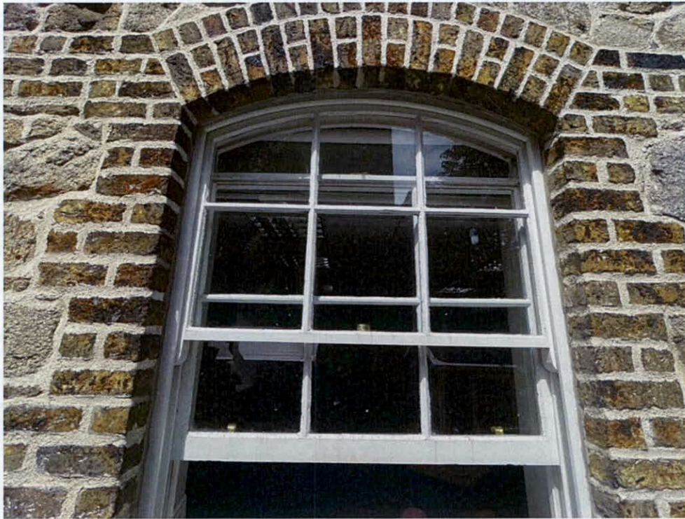
Photo 3: Sample external detail of typical reproduction sash window joinery
