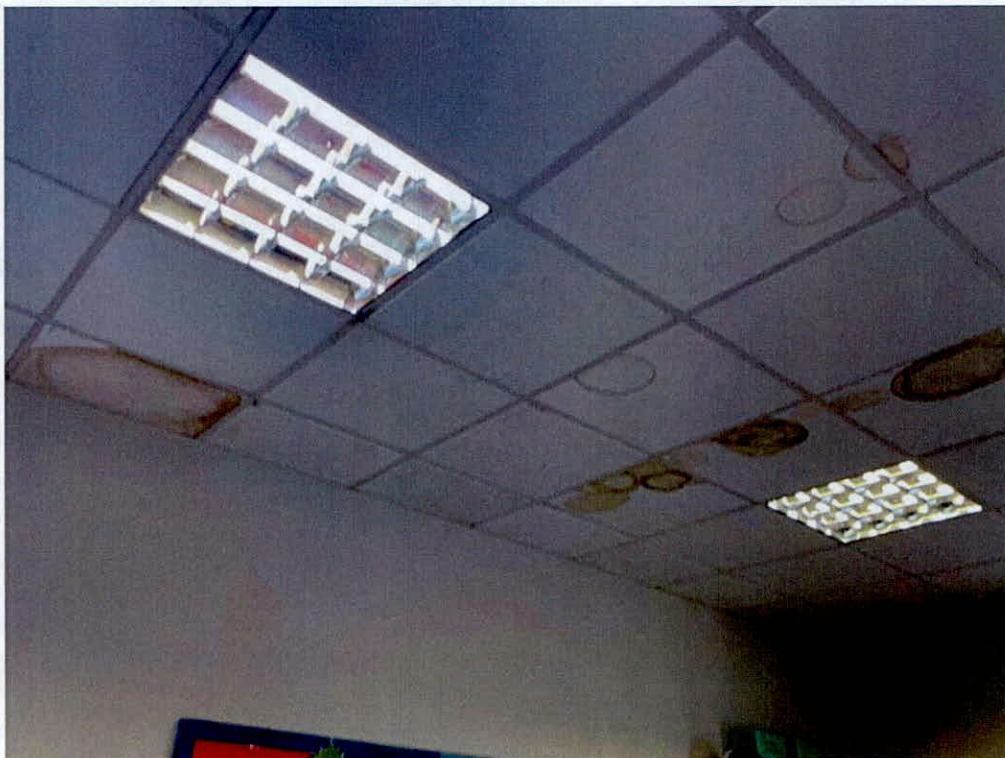
Photo 22: Suspended ceilings and evidence of water ingress
