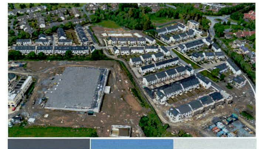
Scholarstown Wood part brick, 2 & 3 storey terraced and semi detached houses and apartments
