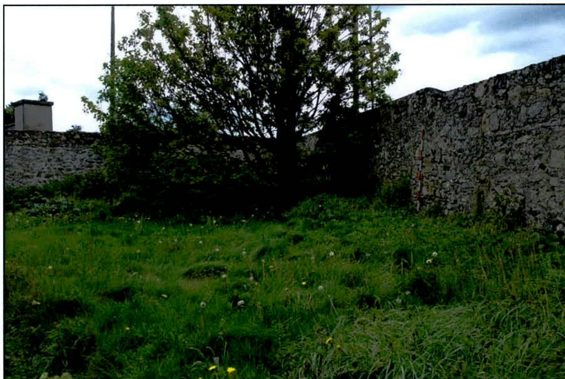
Plate 16 Southern and western walls of walled garden, which also form the property boundary (view to WSW).
