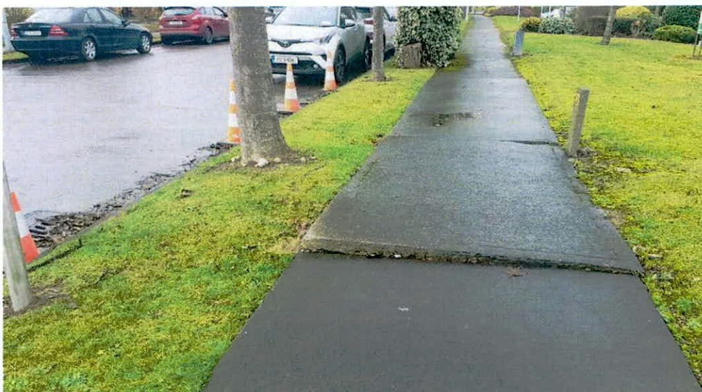
Existing Estate footpath damage due to tree roots (source: SRC)
