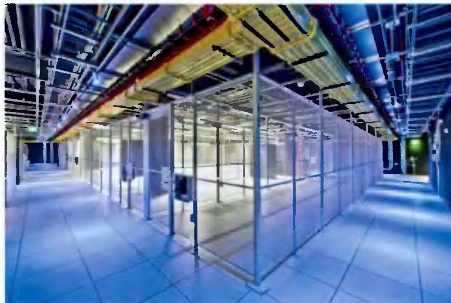
Picture 1: Example of an interior of Equinix Data Centre
