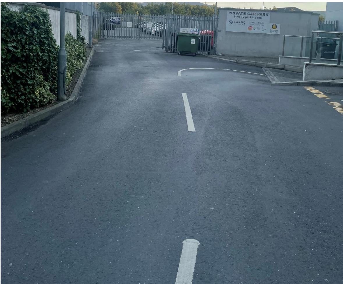
Figure 3 Looking south at the end of the access road where the road drops down to the carpark
