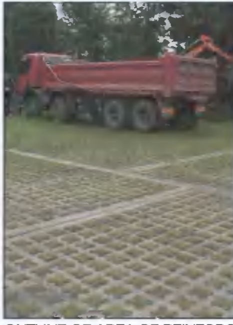
OUTLINE OF AREA OF REINFORCED GRASSCRETE TO FACILITATE TURNING OF FIRE TENDER
