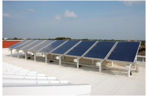
Glazed flat plate collectors
