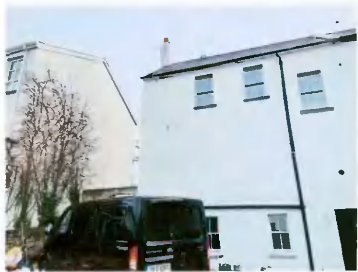
No 14 Rear Facade showing new hardwood sash windows replacing old uPVC with 3 no. existing windows retained and restored
