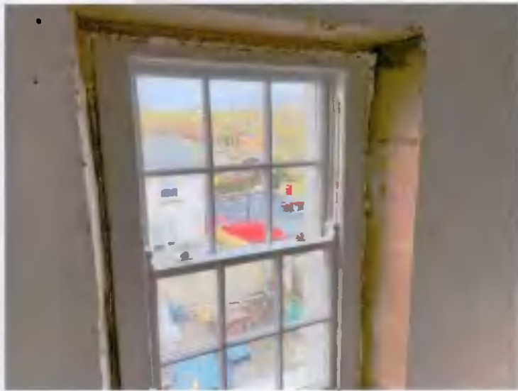
No. 30 First floor - First Floor New hardwood replacement sash window retained to rear
