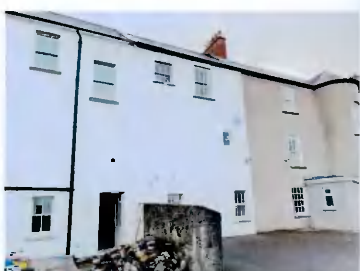
No. 12 Rear Facade showing new hardwood sash windows replacing old uPVC with 3 no. existing windows retained and restored
