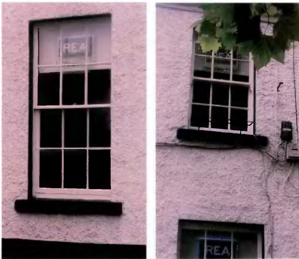
Fig. 10 & 11. Window to No. 2 The Mall. These attractive windows may themselves be replacements for the originals. It is intended to use these windows as models for the replacement of the uPVC windows currently in-situ.
