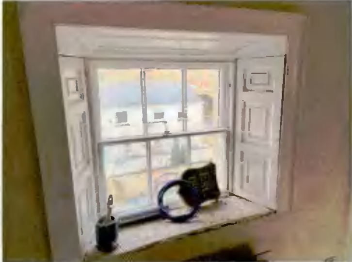
No. 29 First floor - Existing sash window retained and restored with existing original panelling & shutters retained to rear
