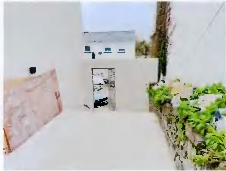
No. 10 Existing modern concrete apron to side area to be altered to facilitate extension
