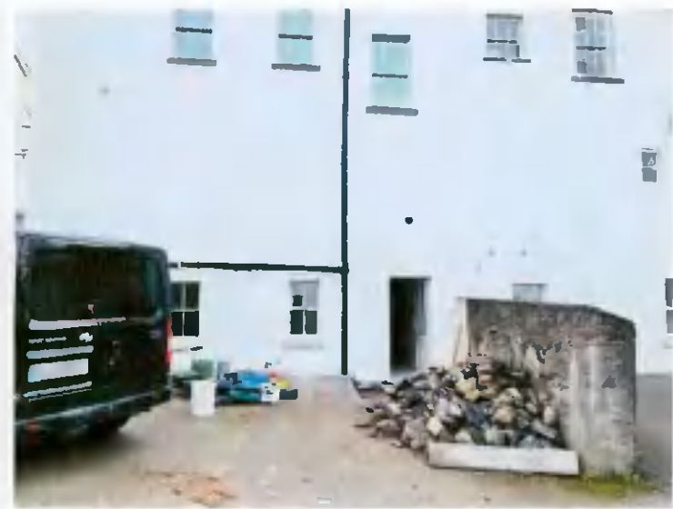
No 13 Rear Facade showing new hardwood sash windows replacing old uPVC with 3 no. existing windows retained and restored
