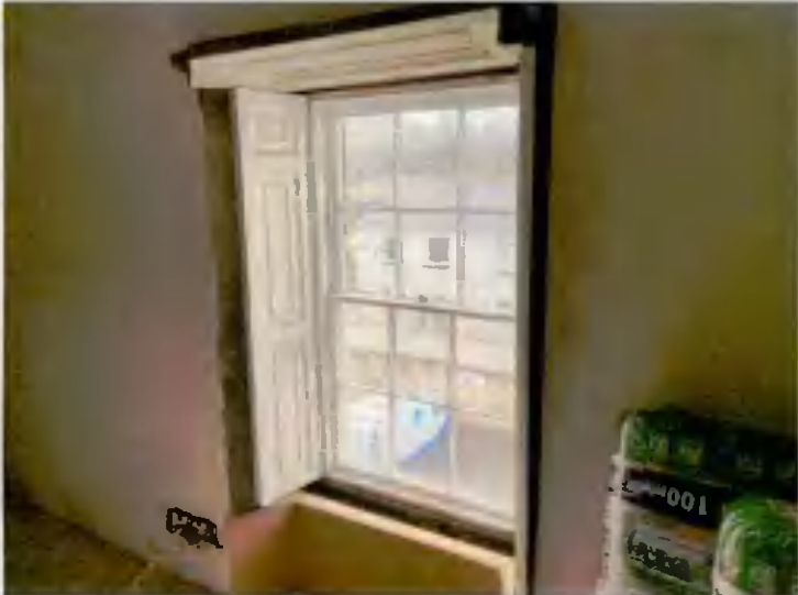
No. 28 First floor - First Floor New hardwood replacement sash window with existing original panelling & shutters retained to rear
