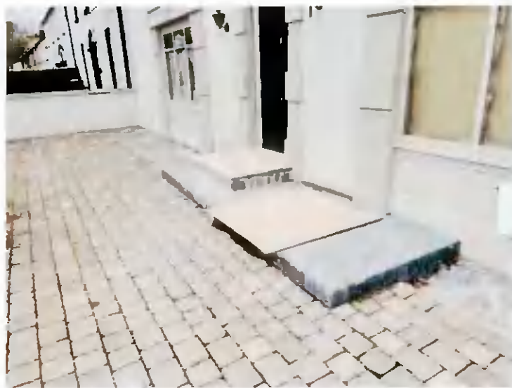
No. 8 Existing Modern entrance steps (to be extended with new ramp provided to facilitate Universal Access)
