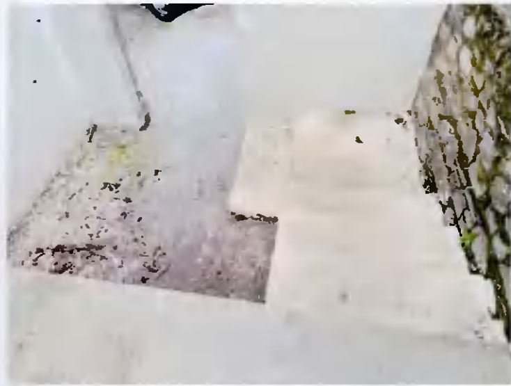
No. 9 Existing modern concrete styeps to side to be removed to facilitate side extension
