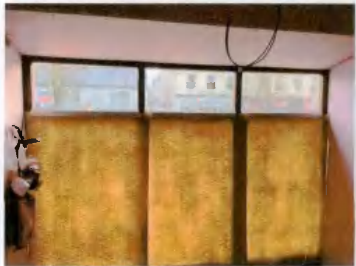
No 26 Ground Floor - view of modern shopfront windows to be replaced & upgraded
