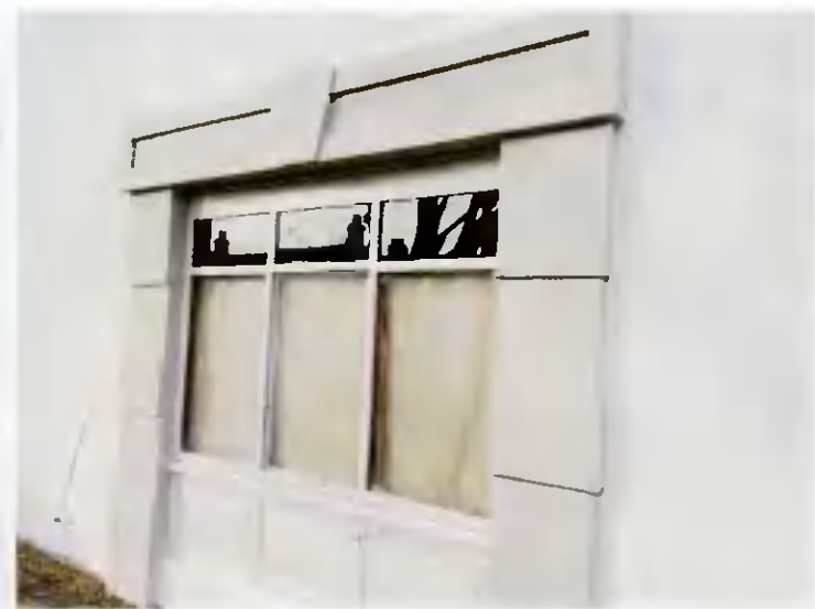
No. 7 Existing front facade with late C.20th modern timber shopfront to be replaced & upgraded (surrounds unaffected)
