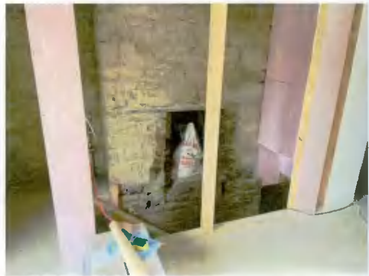
No. 33 First floor - End gable & ex chimney breast with modern stud work to be removed
