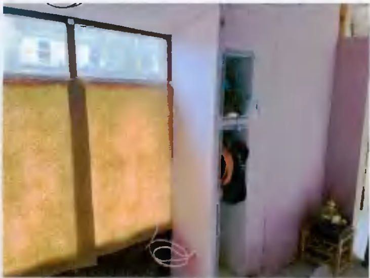
No 25 Ground Floor - view of modern shopfront windows to be replaced & upgraded
