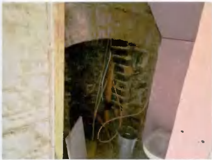
No. 32 First floor - Existing original opening to end gable were new opening proposed, with modern stud work to be removed
