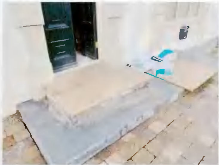
No. 3 Existing Modern entrance steps (to be extended to facilitate Universal Access)
