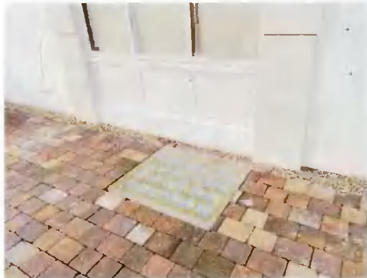
No. 6 Existing front facade with late C.20th modern timber shopfront to be replaced & upgraded (surrounds unaffected) with glass block laylight in ground to bathroom below
