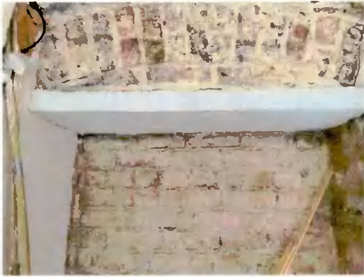
No. 28 First floor - View of gable wall to end gable at rear
