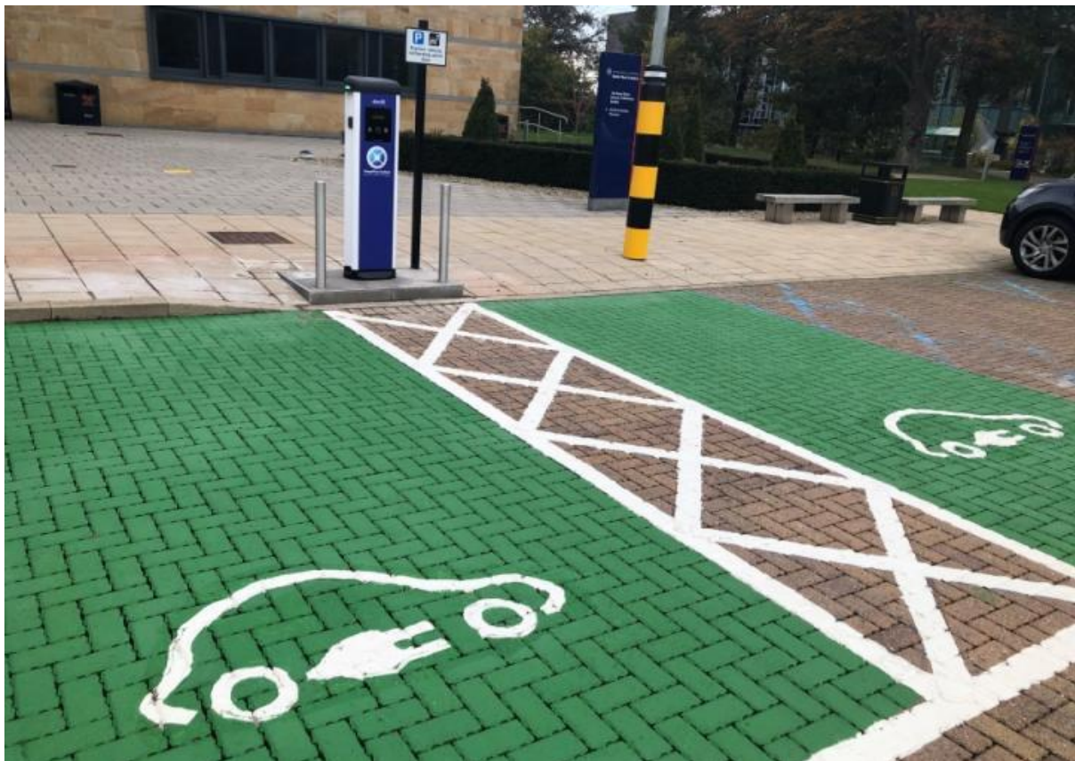
EV Charging Point
