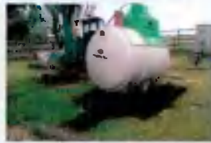
▶ No need for big excavators and large holes that damage your lawn or your garden.
