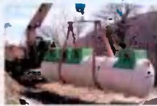
▶ Each unit is made of polyethylene (HDPE) and is made in a way to be easier when transporting the installation blocks.
