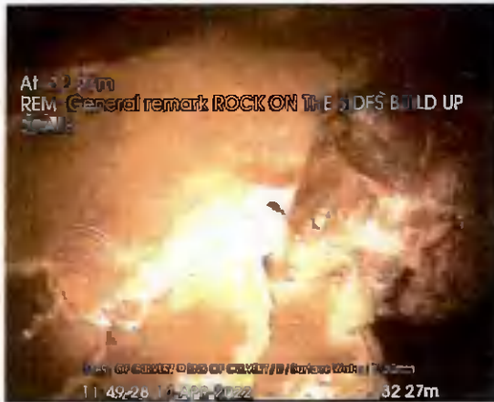
START OF CULVERT US TO END_32-27m_114928.jpg, 00:10:16, 32.27 m General remark, ROCK ON THE SIDES BUILD UP SCALE
