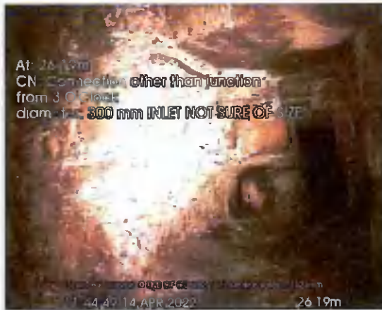
START OF CULVERT US TO END_26-19m_114449.jpg, 00:08:07, 26.19 m Connection other than junction at 3 o'clock, 300mm dia, INLET
