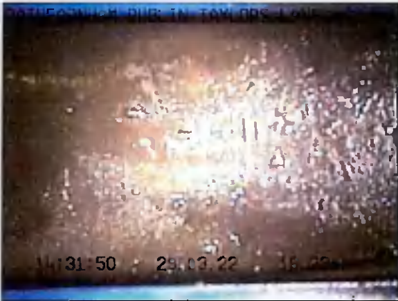
S1.5X_50f16f44-8b2b-41d9-bf27-89650614e110_20220329_143426_104.jpg, 00:02:54, 16.23 m Open joint, large
