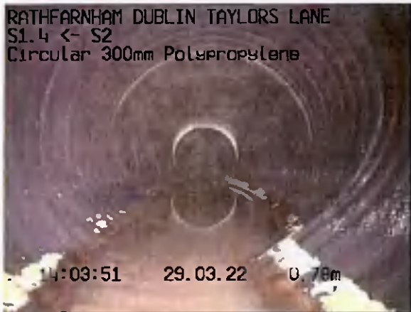
S1.4X_d2016815-55fb-4ec1-a17c-6af5c72a6526_20220329_1 40627_546.jpg, 00:00:21, 0.78 m Deformed sewer or drain, 5%
