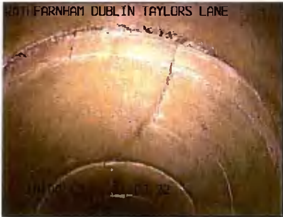
S5X_183cbfbc-eafe-4075-8f26-a2a1f653bb64_20220331_100250_351.jpg, 00:01:28, 4.39 m Fracture, longitudinal at 12 o'clock, start
