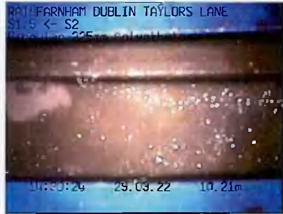
S1.5X_e49f8bd9-b689-4d84-8727-58ddcba34920_20220329_143300_016.jpg, 00:01:55, 10.21 m Open joint, medium
