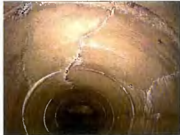
S6X_bc99ee6a-22e3-4f6c-b082-614ea2d5b775_20220330_1 24738_566.jpg, 00:02:45, 13.28 m Crack, longitudinal at 3 o'clock
