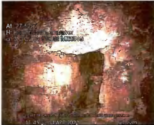
START OF CULVERT US TO END_27-62m_114555.jpg, 00:08:44, 27.62 m Hole in drain or sewer at 3 o'clock, STONE MISSING
