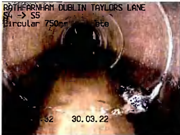
S4X_8730c800-cb5c-41e8-b48b-5606efc9a2ca_20220330_14 5908_327.jpg, 00:01:09, 9.84 m Settled deposits, hard or compacted at joint, 5% cross-sectional area loss
