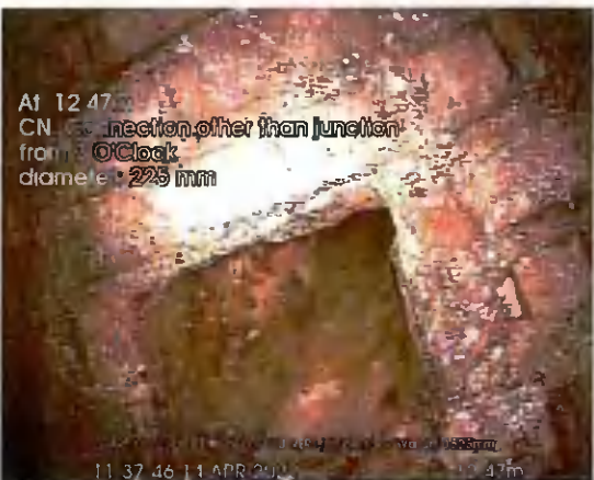
START OF CULVERT US TO END_12-47m_113746.jpg, 00:04:26, 12.47 m Connection other than junction at 3 o'clock, 225mm dia
