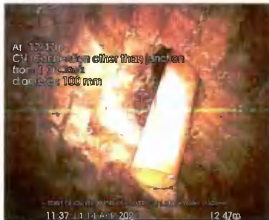
START OF CULVERT US TO END_12-47m_113714.jpg, 00:04:20, 12.47 m Connection other than junction at 1 o'clock, 100mm dia
