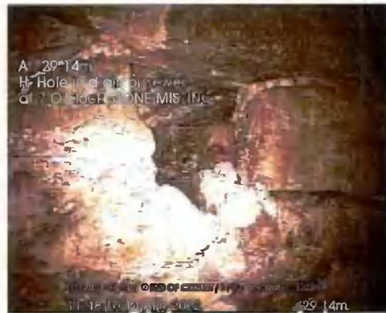
START OF CULVERT US TO END_29-14m_114810.jpg, 00:09:32, 29.14 m Hole in drain or sewer at 7 o'clock, STONE MISSING
