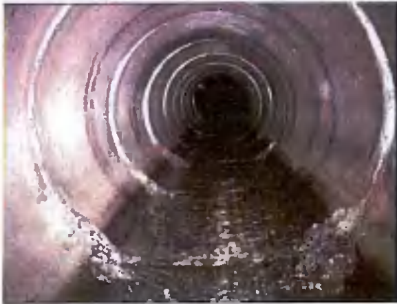
CULVERTX_48eba245-cec1-4feb-a1db-320766e1c5b2_2022 0329_104036_757.jpg, 00:00:42, 0.97 m Settled deposits, hard or compacted at joint, 5% cross-sectional area loss, start
