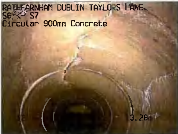
RATHFARNHAM DUBLIN TAYLORS LANE S6X S7 Circular 900mm Concrete S6X_7f8de206-7f78-4a4a-8268-73c4d8761dac_20220330_12 4723_357.jpg, 00:02:42, 13.28 m Crack, longitudinal at 10 o'clock
