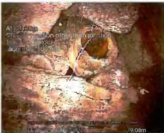
START OF CULVERT US TO END_29-08m_114747.jpg, 00:09:25, 29.08 m Connection other than junction at 11 o'clock, 100mm dia
