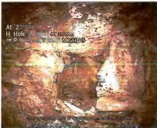
START OF CULVERT US TO END_27-70m_114655.jpg, 00:09:01, 27.70 m Hole in drain or sewer at 9 o'clock, STONE MISSING
