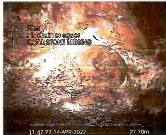
START OF CULVERT US TO END_27-70m_114722.jpg, 00:09:10, 27.70 m Hole in drain or sewer at 7 o'clock, STONE MISSING
