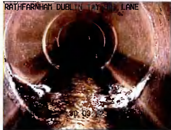
S4X_cbc53040-6ae0-42cf-a44c-890966af4f43_20220330_145 850_844.jpg, 00:00:57, 8.11 m Settled deposits, hard or compacted at joint, 5% cross-sectional area loss
