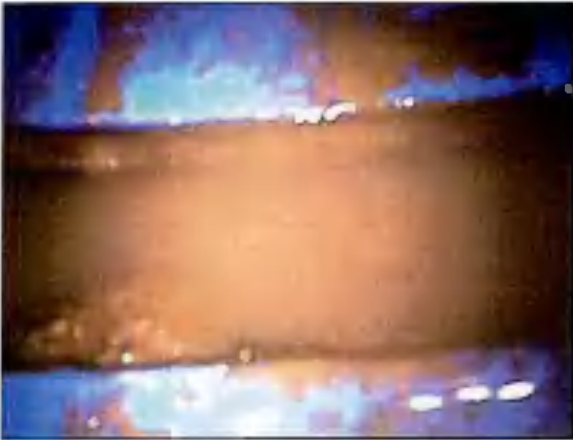
S1.2X_0c58f73f-b250-419b-bd60-b753574c6322_20220329_120551_242.jpg, 00:02:17, 23.43 m Open joint, medium
