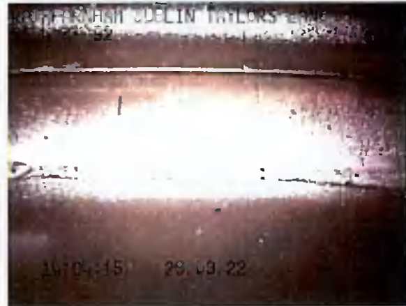
S1.4X_0da55321-7c5d-4ec6-aaa1-ee1b9d635355_20220329 _140650_859.jpg, 00:00:40, 2.96 m Open joint, large
