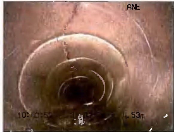
S5X_7dd5fbb8-d536-49ae-93d3-42e36104fe12_20220331_100329_720.jpg, 00:01:53, 4.53 m Crack, circumferential from 9 o'clock to 11 o'clock
