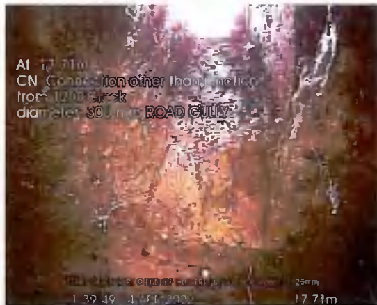
START OF CULVERT US TO END_17-71m_113949.jpg, 00:05:31, 17.71 m Connection other than junction at 12 o'clock, 300mm dia,
