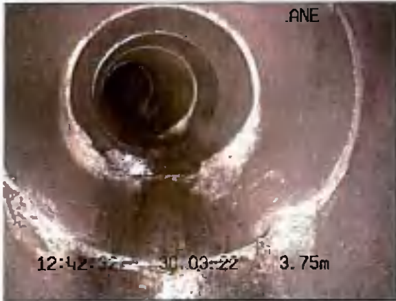
S6X_2c89ba3a-d39c-4a24-869f-47e9db03a731_20220330_1 24509_496.jpg, 00:00:53, 3.75 m Settled deposits, hard or compacted at joint, 5% cross-sectional area loss, start
