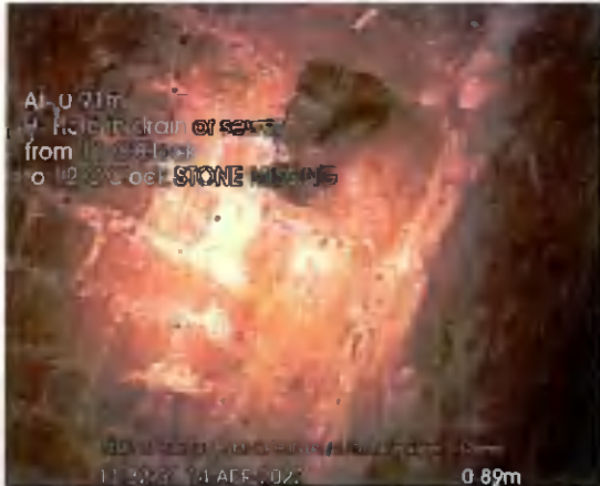
START OF CULVERT US TO END_0-89m_113251.jpg, 00:00:45, 0.89 m Hole in drain or sewer from 11 o'clock to 12 o'clock, STONE
