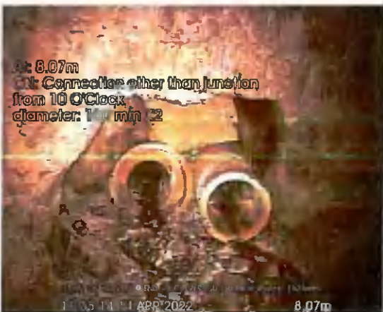
START OF CULVERT US TO END_8-07m_113514.jpg, 00:02:29, 8.07 m Connection other than junction at 10 o'clock, 100mm dia, X2
