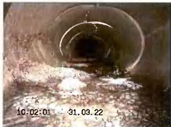
S5X_a89bf5fe-b788-48ab-b650-d55207f2059_20220331_100438_511.jpg, 00:02:25, 6.15 m Roots, mass, 25% cross-sectional area loss, start, ROOTS
