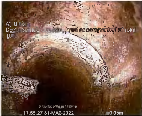
G2 DS S4_0-06m_115527.jpg, 00:00:05, 0.06 m Settled deposits, hard or compacted at joint, 10% cross-sectional area loss
