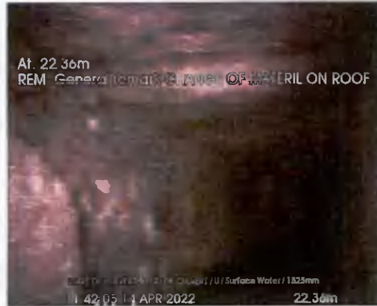
START OF CULVERT US TO END_22-36m_114205.jpg, 00:06:51, 22.36 m General remark, CHANGE OF MATERIL ON ROOF
