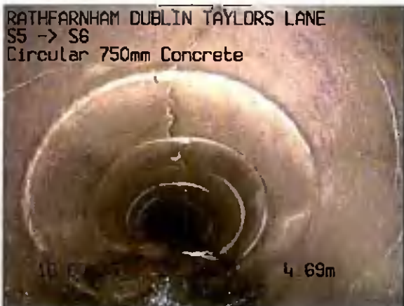
S5X_70bcc9d2-7e16-46d6-ac68-2d55e5bc361e_20220331_100312_436.jpg, 00:01:42, 4.69 m Crack, circumferential from 2 o'clock to 4 o'clock
