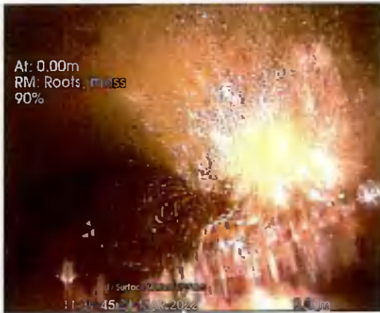
S5 US LINE2_0-00m_113945.jpg, 00:00:02, 0.00 m Roots, mass, 90% cross-sectional area loss
