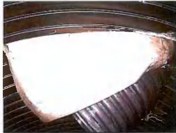
CULVERTX_e39f477b-5958-4e6a-b631-86e679e6465d_2022 0329_104457_213.jpg, 00:02:30, 11.48 m General remark, ROCK INTRUDING INTO PIPE
