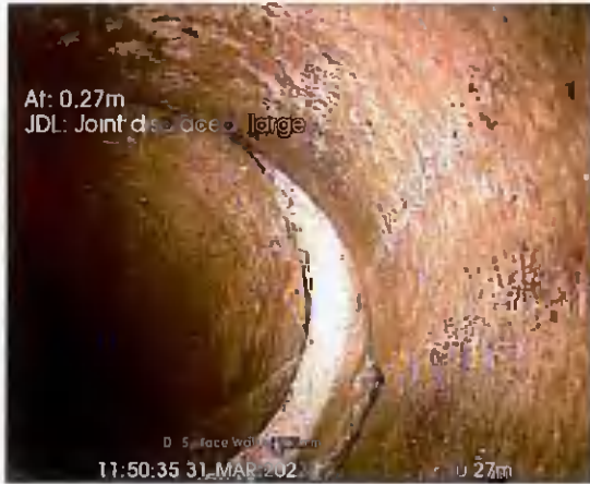
G1 DS S4_0-27m_115035.jpg, 00:00:07, 0.27 m Joint displaced, large
