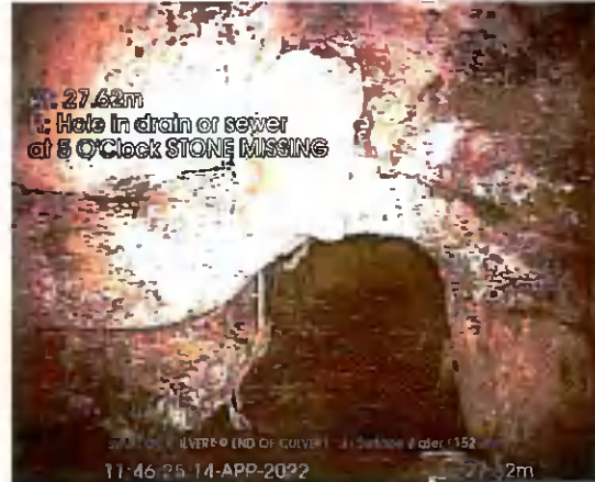
START OF CULVERT US TO END_27-62m_114625.jpg, 00:08:49, 27.62 m Hole in drain or sewer at 5 o'clock, STONE MISSING
