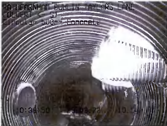
CULVERTX_a9b2f890-dc0d-4c0c-8ca4-898a1a8e911e_20220 329_104225_728.jpg, 00:01:39, 10.14 m Connection defective, connecting pipe is intruding at 2 o'clock, 225mm dia, intrusion: 15%
