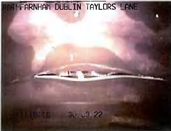
S1.6X_1baee87f-36f9-4e0f-b874-52db4dacc49b_20220330_1 12052_465.jpg, 00:09:08, 76.18 m Hole in drain or sewer at 12 o'clock
