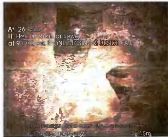
START OF CULVERT US TO END_26-15m_114405.jpg, 00:07:49, 26.15 m Hole in drain or sewer at 9 o'clock, STONE MISSING 2
