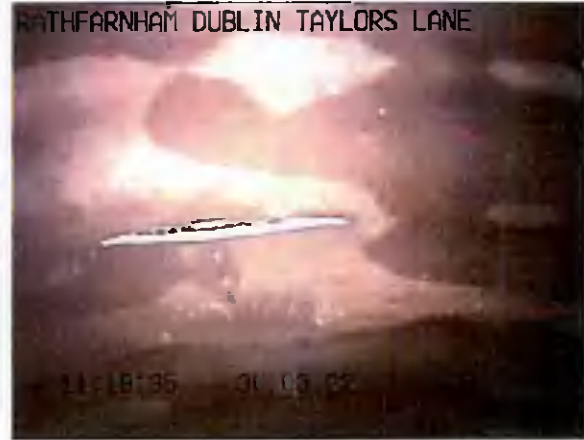
S1.6X_0c42c29f-49f0-4671-9a28-23decd23b8fc_20220330_1 12110_822.jpg, 00:09:20, 76.34 m Hole in drain or sewer at 12 o'clock
