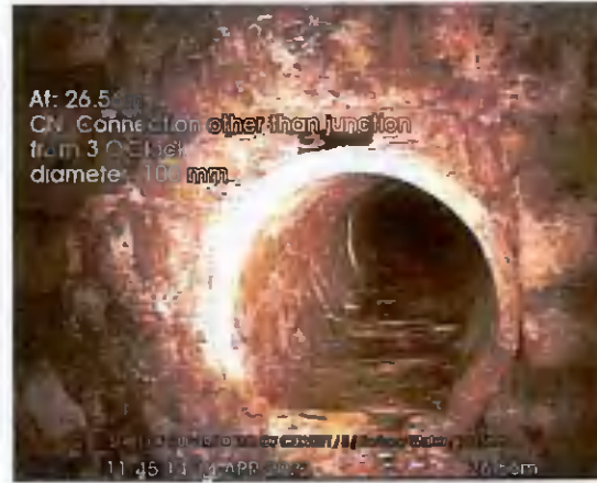
START OF CULVERT US TO END_26-56m_114514.jpg, 00:08:22, 26.56 m Connection other than junction at 3 o'clock, 100mm dia
