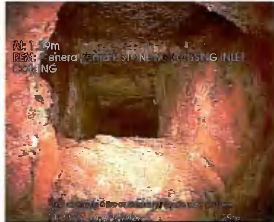
START OF CULVERT US TO END_1-29m_113327.jpg, 00:00:55, 1.29 m General remark, STONE NOT MISSING INLET COMING
