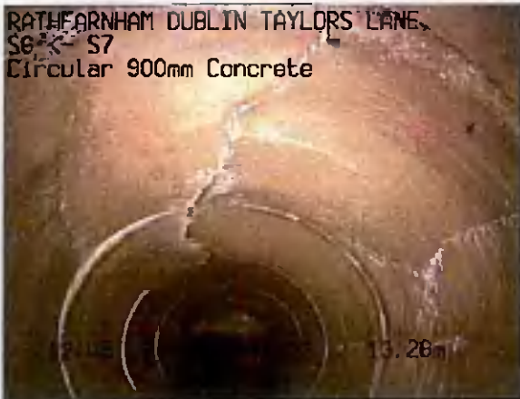
S6X_5c0d0b39-e48c-4253-82f3-0e5c4f26af42_20220330_124752_449.jpg, 00:02:49, 13.28 m Crack, longitudinal at 4 o'clock
