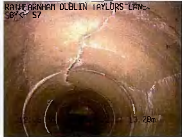
S6X_7eb2e6a5-88f2-4002-b479-51d6eb647213_20220330_124806_940.jpg, 00:02:53, 13.28 m Crack, longitudinal at 12 o'clock, start
