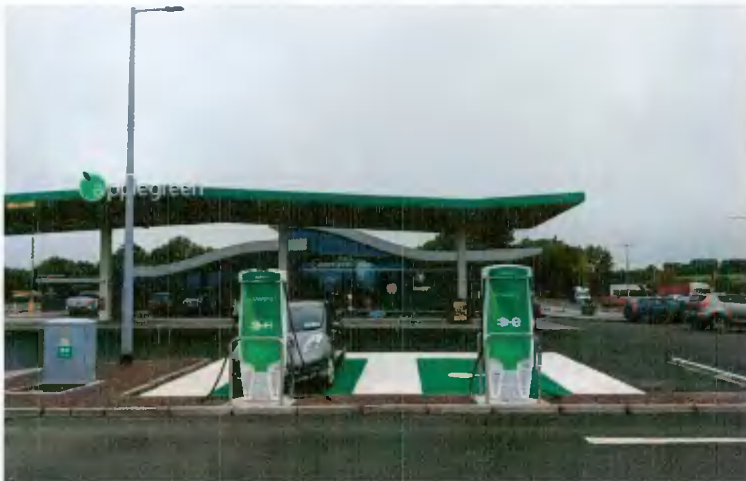
Fig No.5 Typical example of Applegreen EV Chargers located in Birdhill, Co Tipperary
