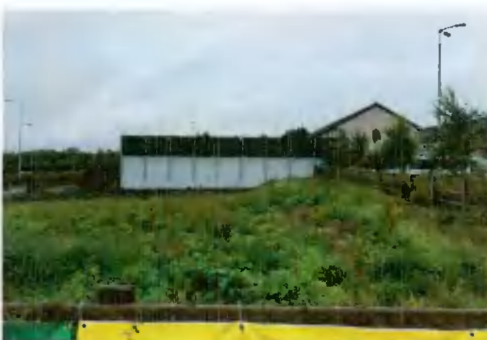
Fig No.4 Photograph from west end of site facing east showing large retaining wall and fencing over along eastern boundary.
