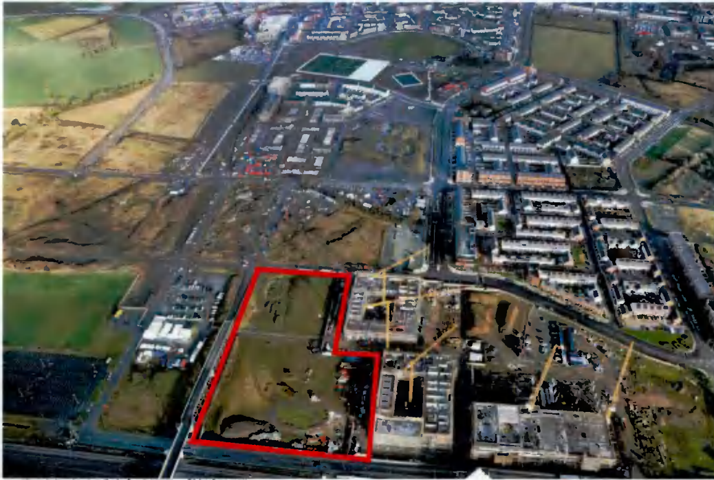
Figure 2: Aerial Photograph of the Adamstown Station tile and its immediate environs on 4 th February 2022 showing progress of the construction of Blocks B, E and F (Phase 1 at The Crossings). Outline of application site shown approximately in red. (source: Barrow Coakley Photo & Video)
