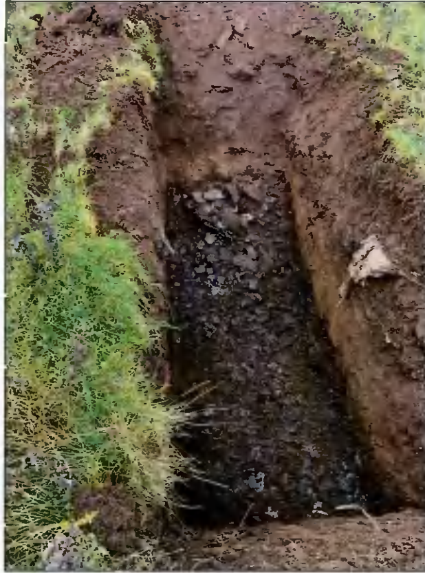
Plate 9 T3P 1.2m wide x 3m long, revealed fill material, excavated to 1.8m in depth
