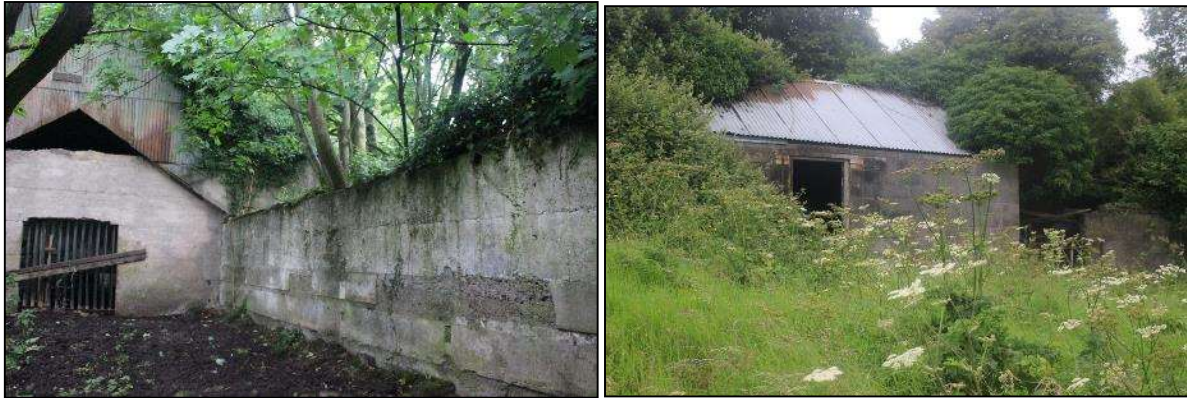
Plates 1 & 2 - Cattle shed in the south east of the site (left) and intact building in the south west of the site (right)
