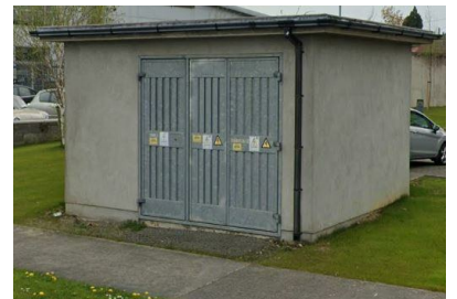
IMAGE OF STANDALONE SUB STATION TO ESB SPECIFICATIONS
