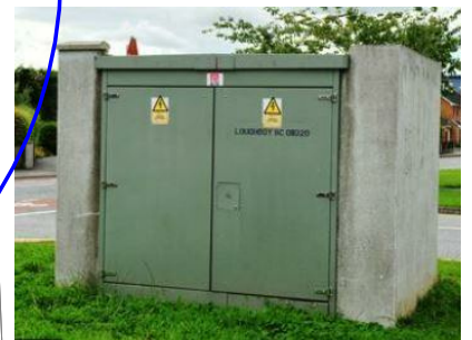
IMAGE OF TYPICAL UNIT STANDALONE SUB TO ESB SPECIFICATIONS
