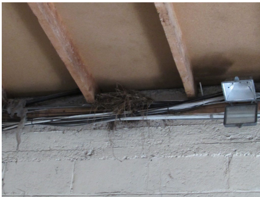
Figure 5-10. Feral pigeon nest within a warehouse at the Proposed Development Site.
