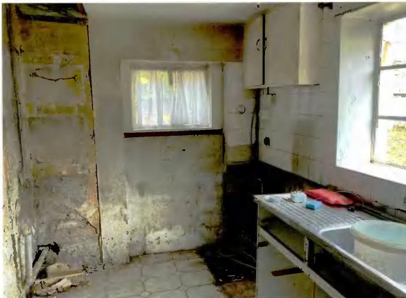
Above: The direction of the ceiling joists over the corner extension basement room is visible in the top left corner.
