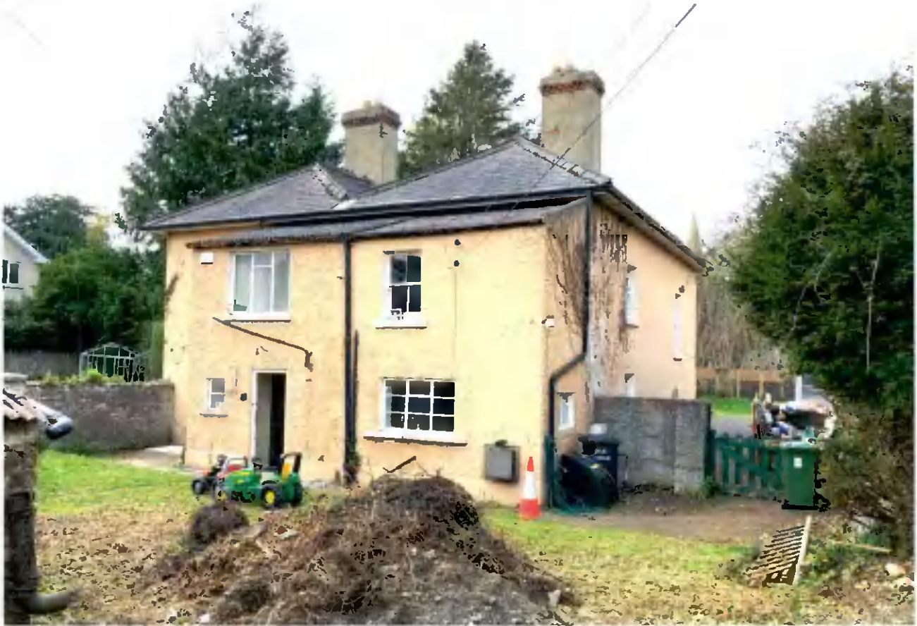
Above: Asbestos roofed extension proposed for demolition & slated corner extension to be retained.
