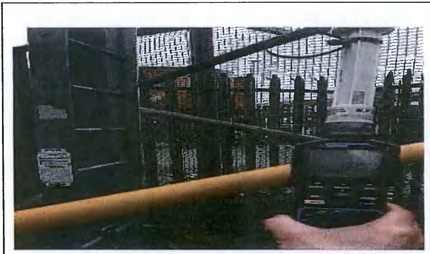
RF Emissions Reading No.2 Photograph
