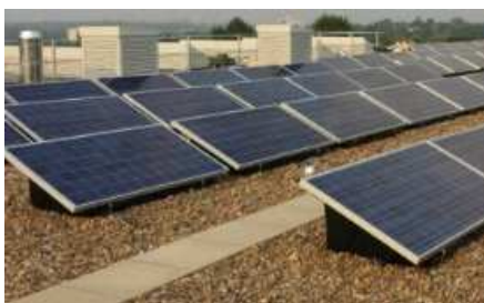
Image above of Solar PV Array
