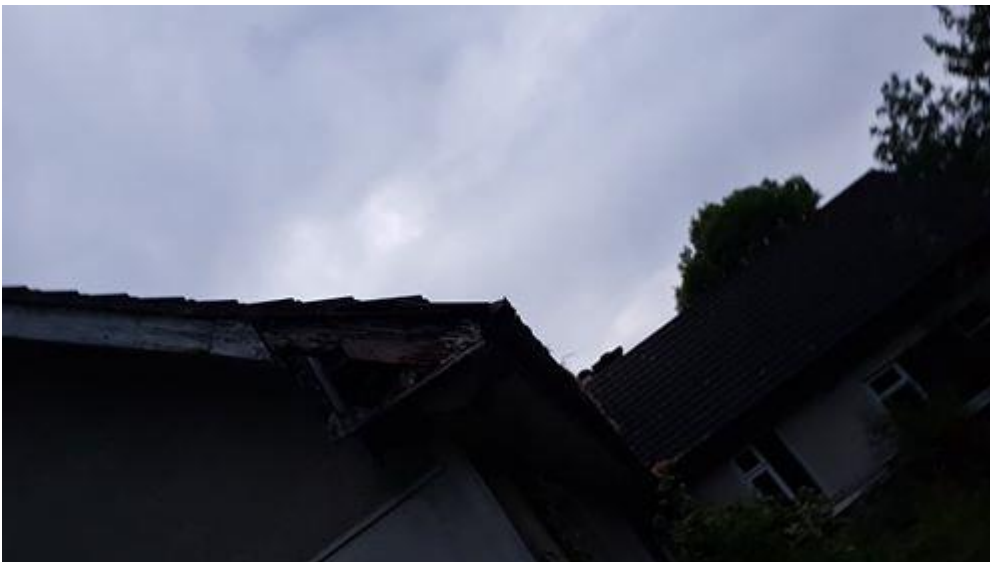
Damage to fascia board would allow bat access
