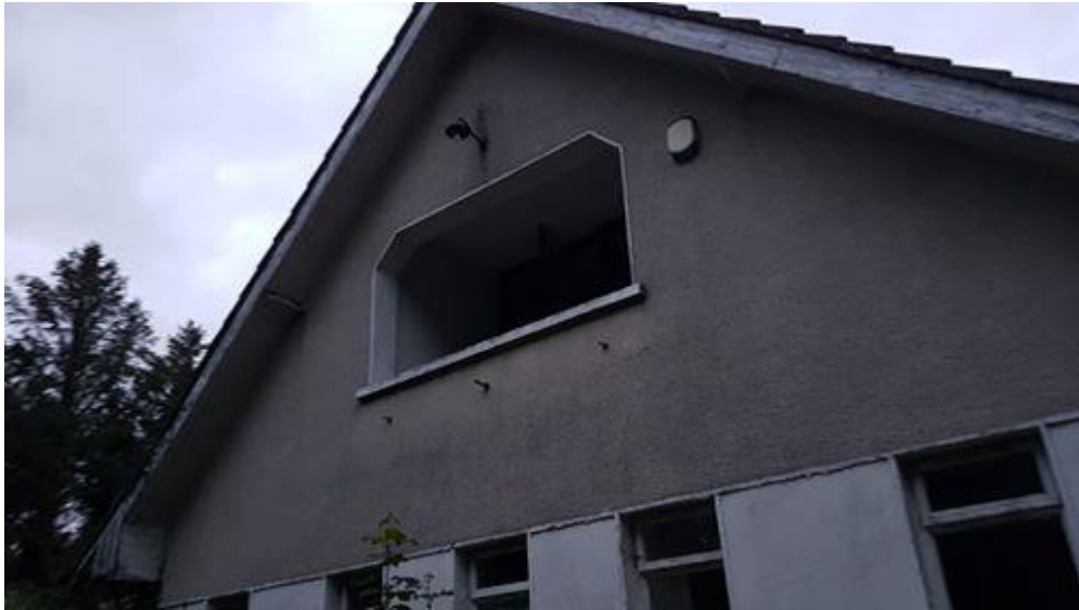
Open windows upstairs allow bat access
