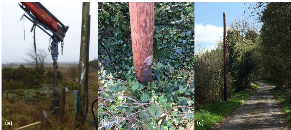
FIGURE 3. (A) UTILITY TRUCK MOUNTED AUGER EXCAVATING HOLE FOR UTILITY POLE, (B) AND (C) NEWLY INSTALLED UTILITY POLES.
