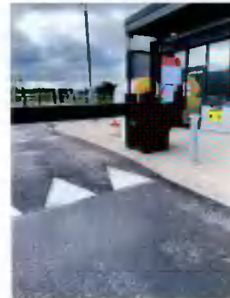
PHOTO No.05 EXISTING HEAVY DUTY TRAFFIC ARM AND CAGE TO BE REMOVED
