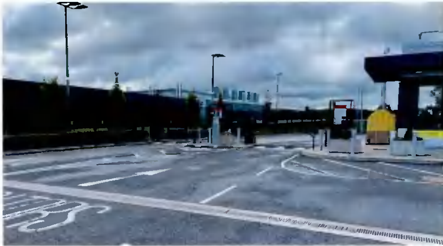
PHOTO No.01 2 NO. APPROACH LANES PROPOSED TO BE WIDENED. POSITION OF NEW TRAFFIC ISLAND AND PROPOSED NEW TRAFFIC ARM TO ALIGN WITH KIOSK ISLAND AND ROAD MARKINGS. SEE ENCLOSED DWG IE0313027-30- DR-0010
