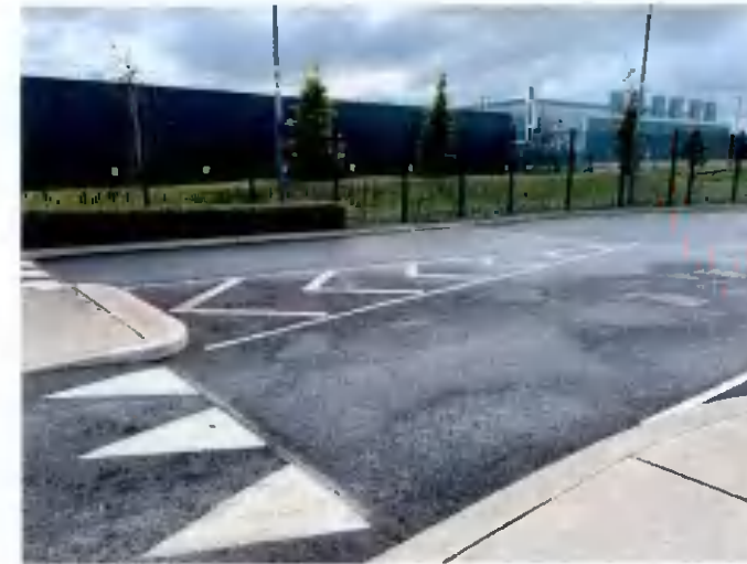
PHOTO No.04 CENTRAL RAISED ISLAND AND ROAD MARKINGS TO BE REMOVED. PROPOSED ROAD BLOCKER AND ROAD MARKINGS TO BE ADDED IN TO THIS LOCATION. SEE ENCLOSED DWG IE0313027-30- DR-0010
