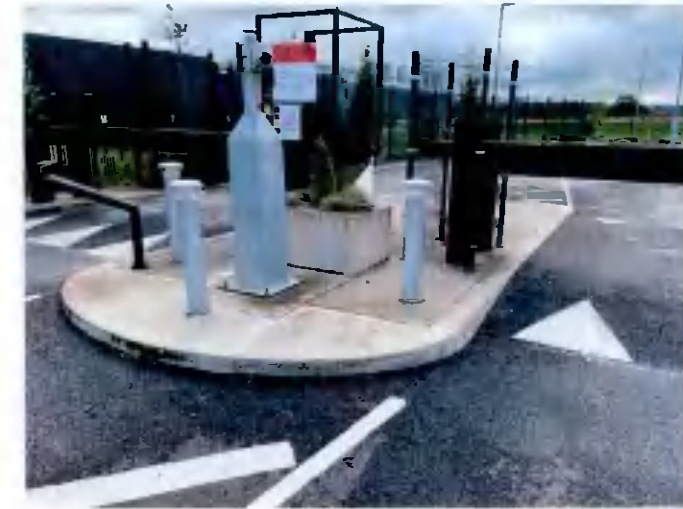
PHOTO No.02 CENTRAL RAISED ISLANDS, BOLLARDS & HEAVY DUTY TRAFFIC BARRIERS TO BE REMOVED
