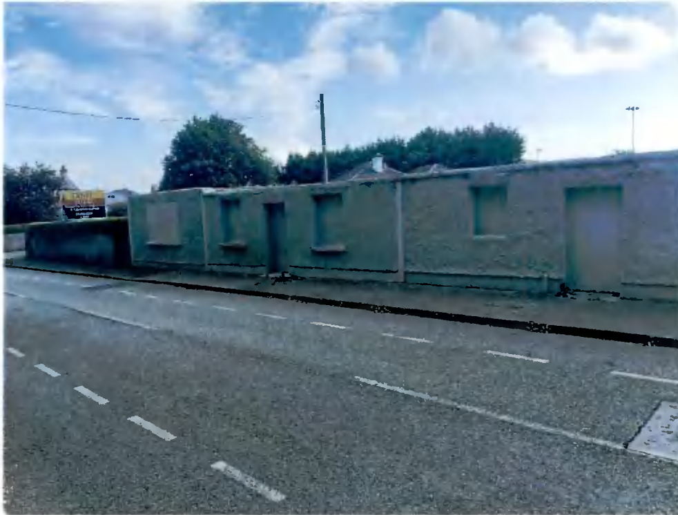
Plate 5: Ruined cottages as viewed from the road, facing northeast
