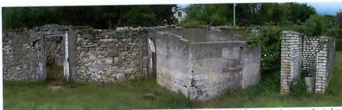
Figure 43 – The rear wall boundary wall of the first northerly cottage with ruined 20thC extensions in concrete (centre) and brick (right) the back door is in the rubble wall.
