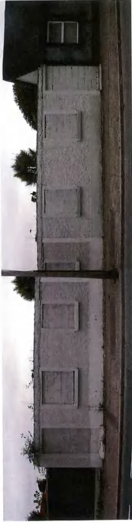
Fig. 8. View of boundary wall double façade adjoining remaining cottage on Whitechurch Road. (C2/3)
