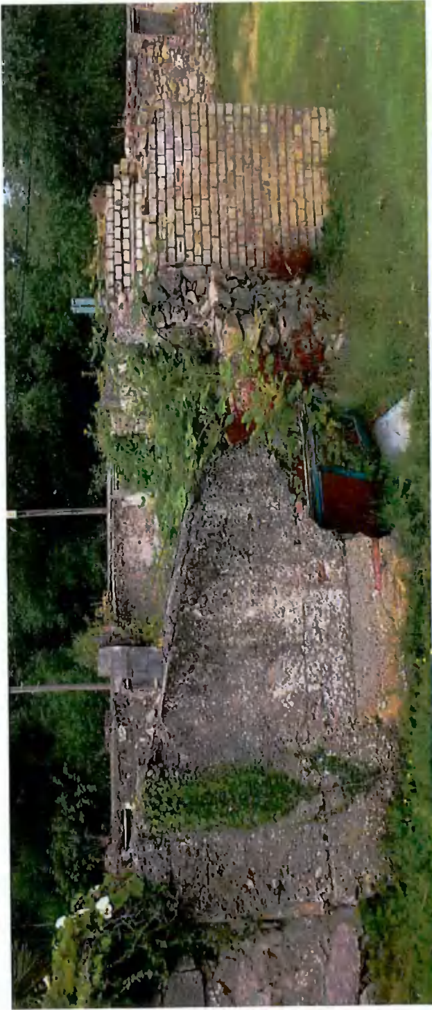
Fig. 46 – View of concrete section of rear garden boundary wall of remaining cottage. (C3)
