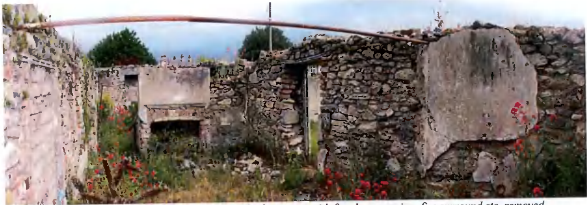
Figure 46 – The gable wall of the first northerly cottage with fireplace opening, fire surround etc. removed.
