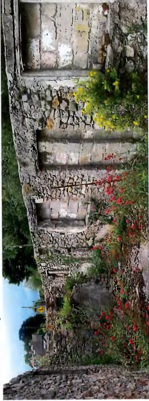
Fig. 54 – View south in north section of middle ruin interior with blocked up openings to Whitechurch Road. (C6)
