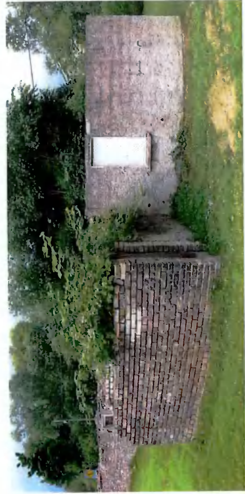
Fig. 49 & 50 – Views of 20thC ruin brick/ concrete walls along west boundary/ along Whitechurch Road. (C6)
