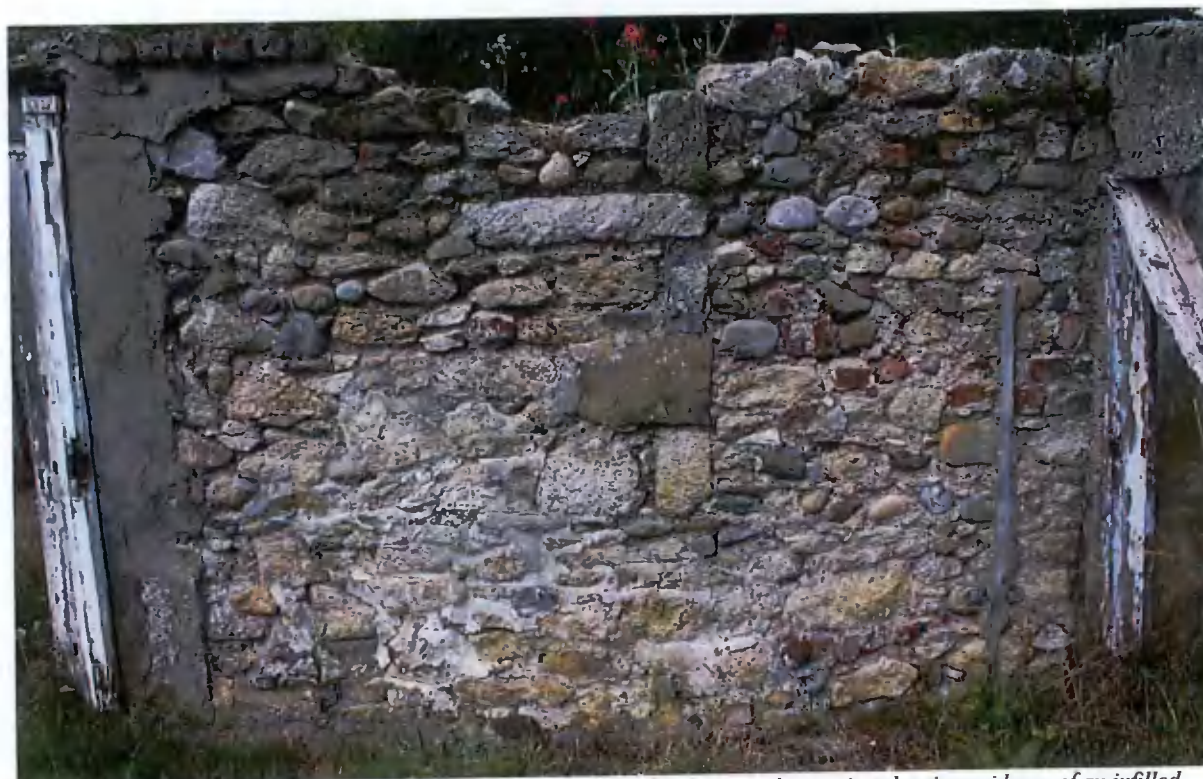
Figure 44 – The original walls are random rubble/ likely local fieldstone, this section showing evidence of an infilled window or door ope. The construction is basic vernacular and unlikely to have any foundation.
