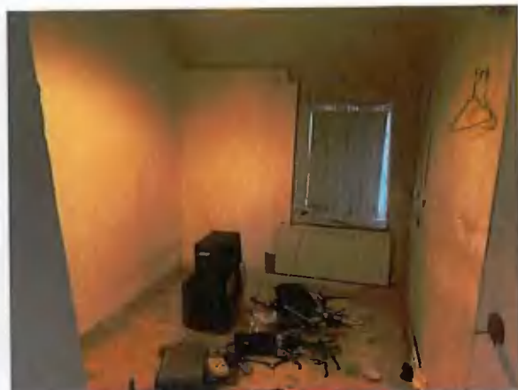
Fig. 32 Dilapidated bedroom in cottage.
