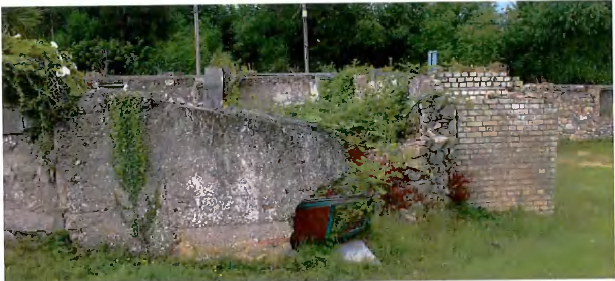
Figure 409 – The rear wall boundary wall of the remaining cottage (6) adjacent to fifth (right). The walls are concrete with some rubble stone and on the fifth a 20thC outside toilet was built in late 20thC brick.
