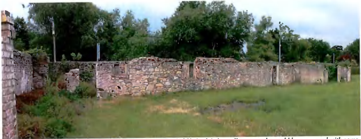
Figure 41 – The rear wall boundary wall of the cottages 1-5, fifth (right) the walls are random rubble uncoursed with some 20thC extensions in brick/ concrete in a similar ruinous condition. The rubble walls would not typically have foundations
