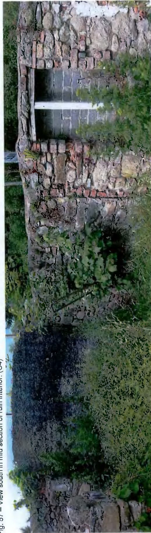
Fig. 58 – View south in south mid section of ruin interior with blocked up openings to Whitechurch Road. (C4)
