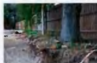
Potential loss of existing tree due to poor construction techniques.
