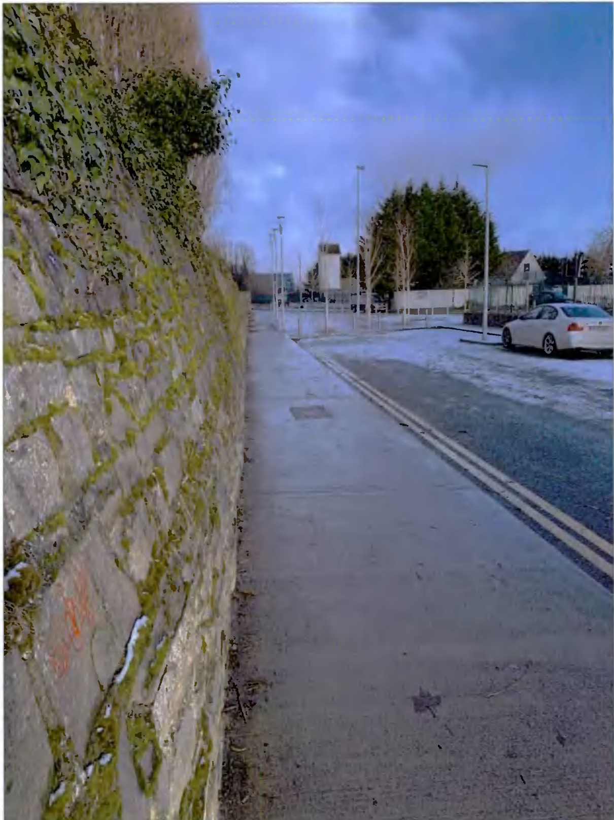
Plate 12: View (north-east) along the outer face of the boundary wall – note the pronounced inward lean at less than one-metre above pavement level
