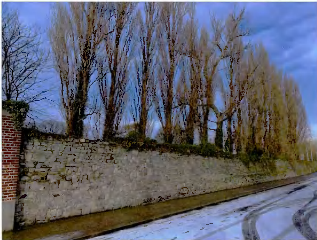
Plate 11: View of the exterior face of the boundary – the poplar trees are planted very close to the wall and appear to have led to significant distortion in the wall itself.
