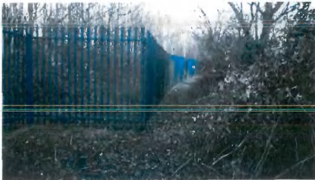
General condition of perimeter fence at western edge of proposed generator yard.
