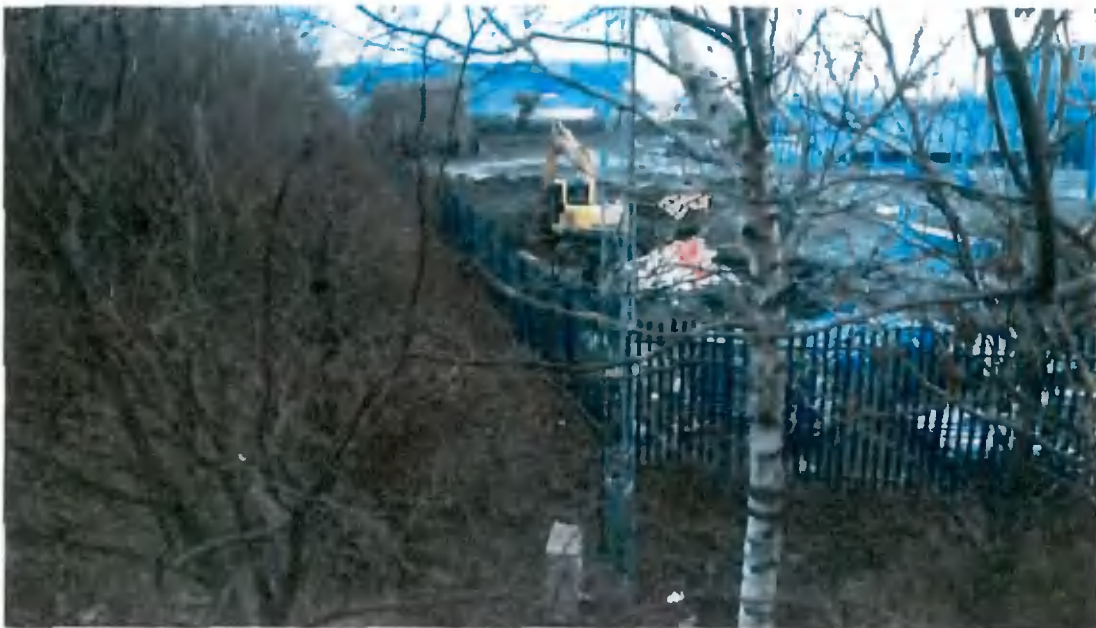
Location of Camera 1 on Takeda site at south east corner of generator yard .
