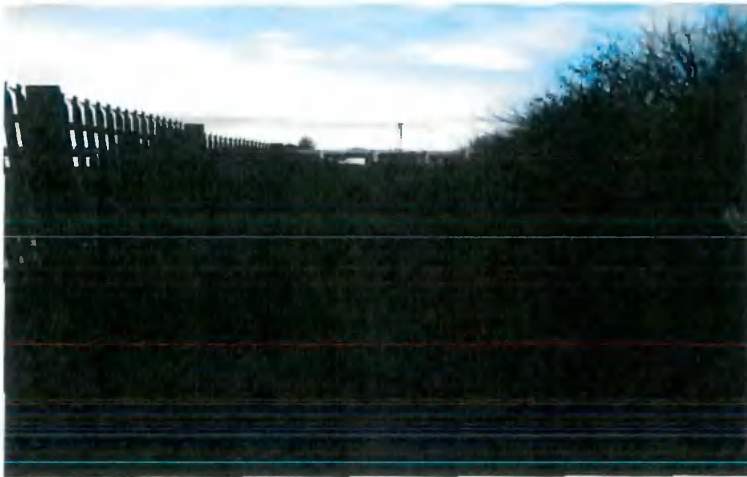
Perimeter fence between Edgeconnex and Takeda site along southern perimeter of generator yard indicating misalignment of fencing
