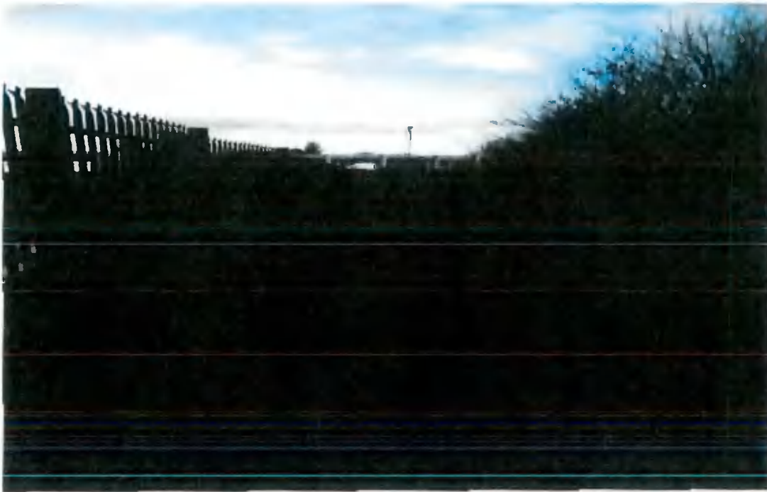
Perimeter fence between Edgeconnex and Takeda site along southern perimeter of generator yard indicating misalignment of fencing
