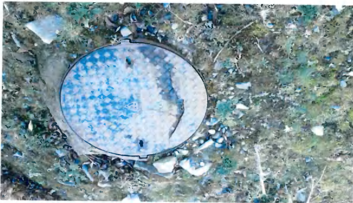
Damaged manhole within Takeda site at north east corner of proposed generator yard.
