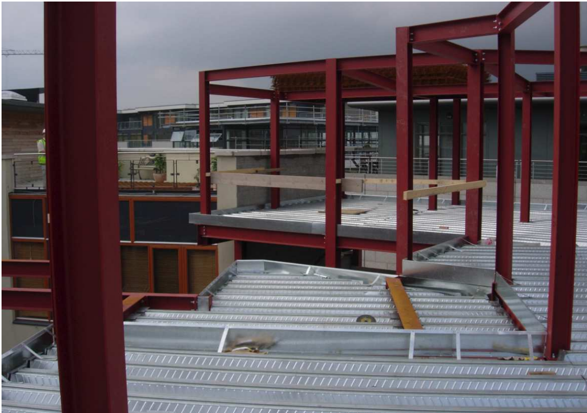
Figure 9: new steel framed building with composite concrete metal deck floors under construction
