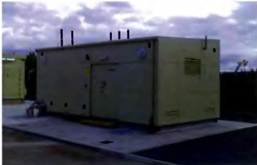
Figure 2 - Typical Boiler/Generator Kiosk
