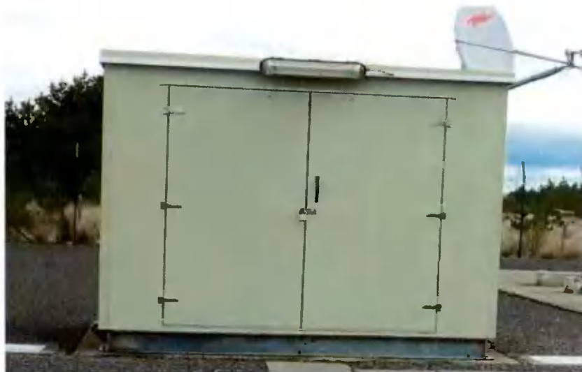
Figure 3 - Typical Electrical/Instrumentation Kiosk
