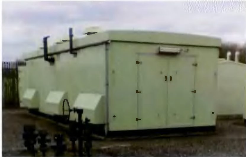
Figure 1 - Typical Regulator/Meter Kiosk
