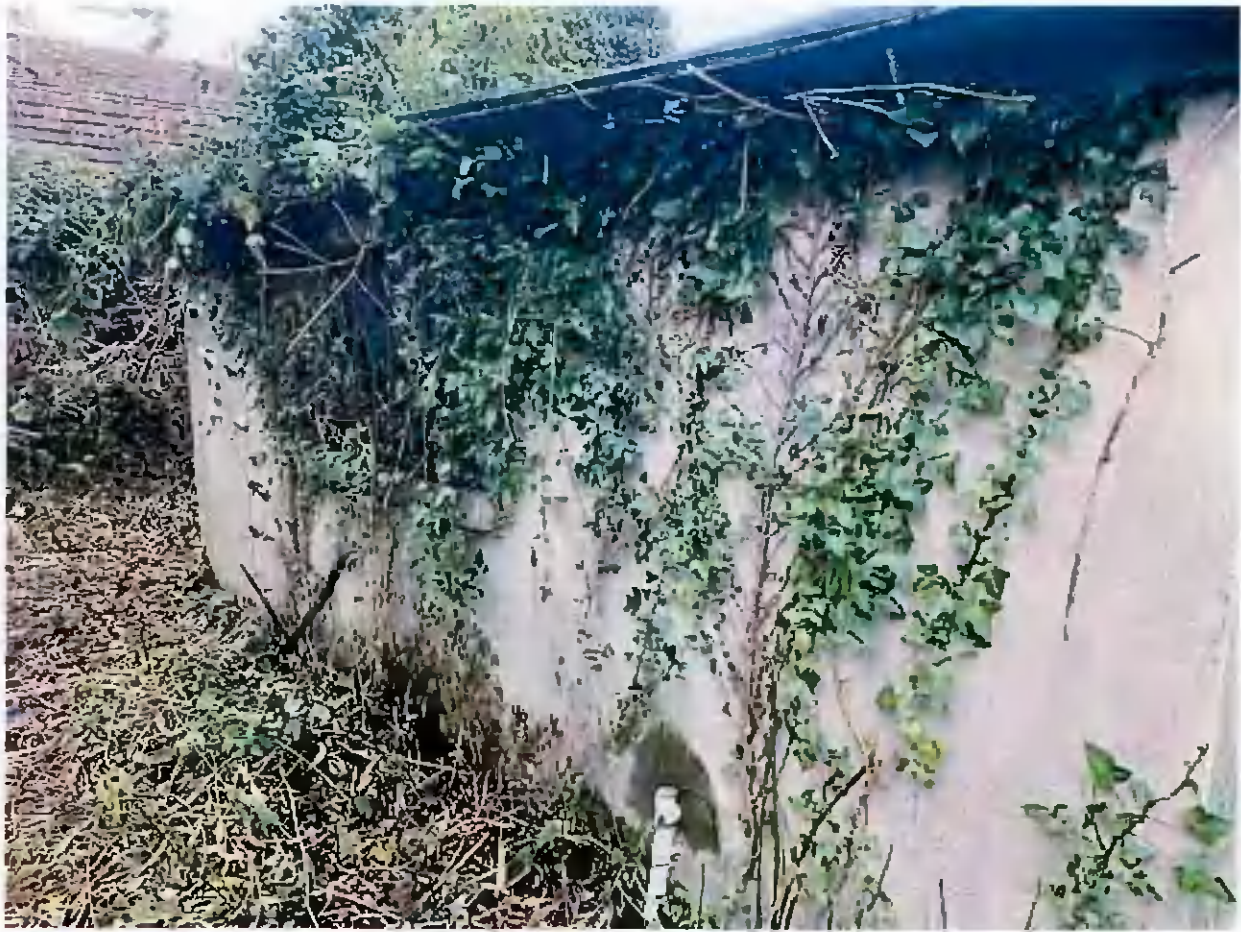
South west corner. Significant vegetation damage at roof edge.
