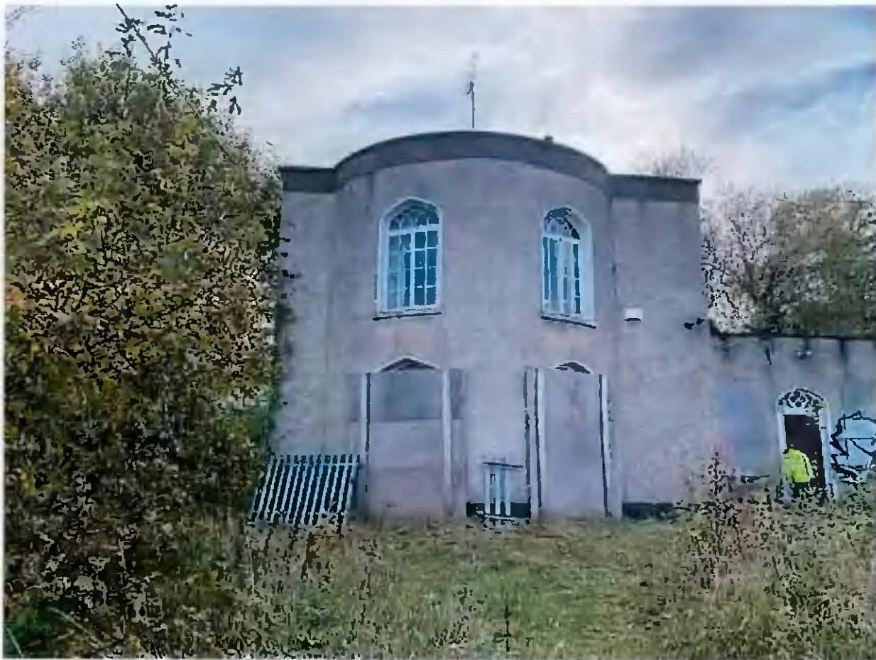
Eastern half of north elevation. Note crack running through left hand window on drum.
