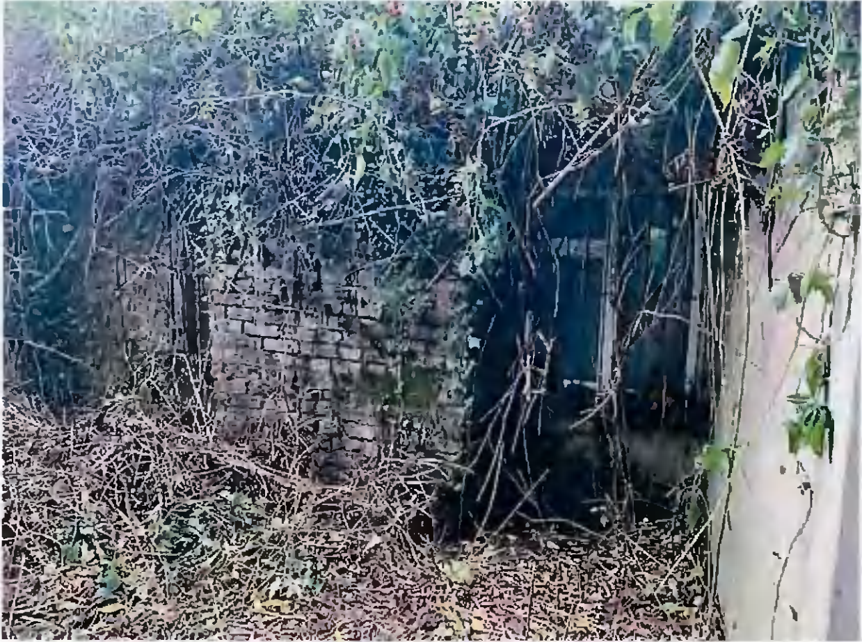
West Rear Corner Overgrown with vegetation
