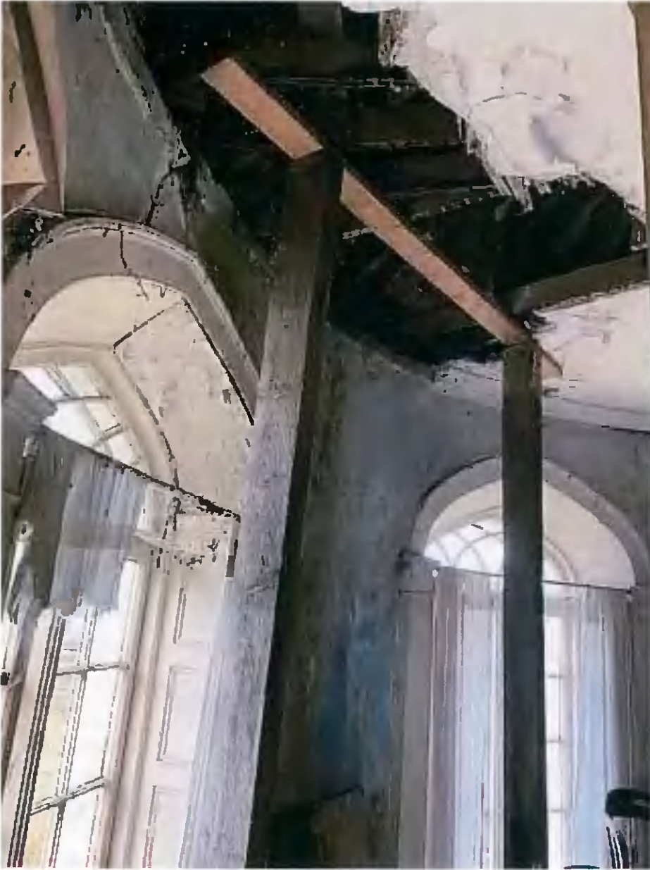
First Floor North Wall Behind Drum Windows and surrounds which should be saved if possible. Note timber propping suggesting significant rotten joist ends putting the saving of the roof structure in doubt.
