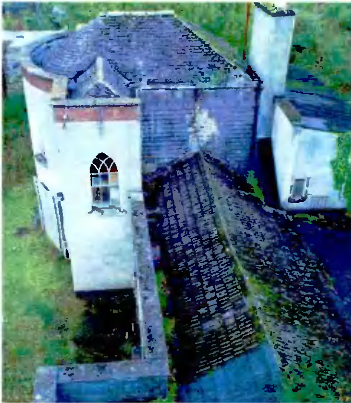
View of bowing tile roof with missing vertical slates beyond
