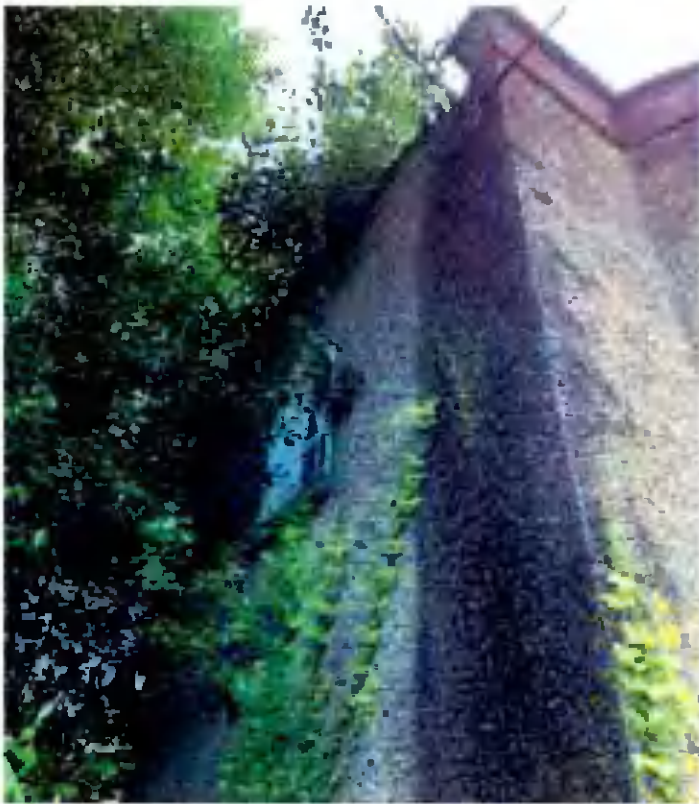
View of eastern damp wall where water is running down wall from parapet gutter
