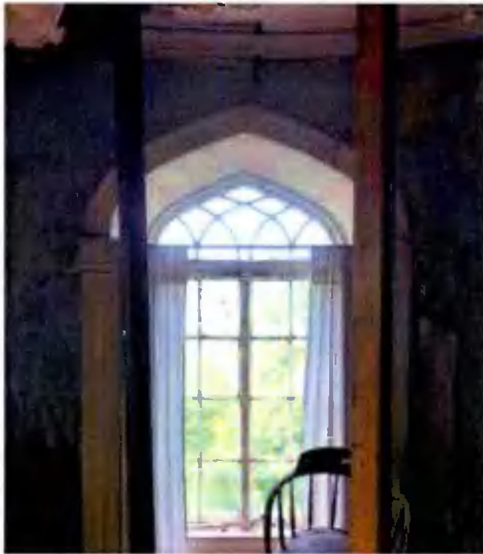
Internal view showing damaged plaster and intact window
