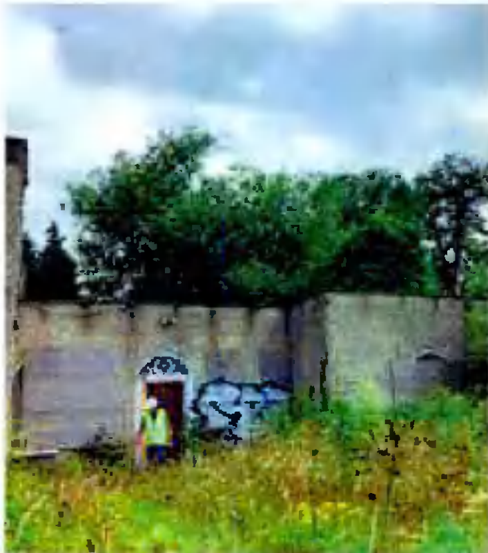
Photo of front of building showing streaks on render below parapet joints
