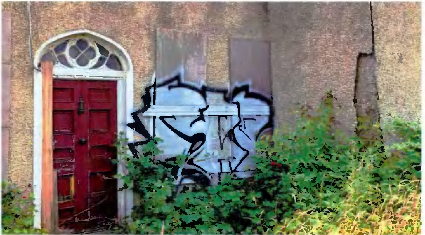
Existing panelled front door and graffiti and bessed render
