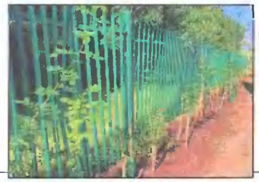
Boundary Type D New native hedgrows and existing fence as permitted under planning permission SD18A/0126. Fence installed prior to 2012 before the applicant acquired the site
