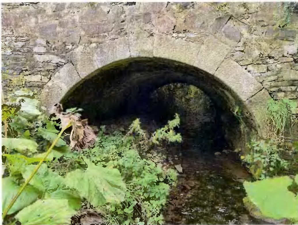
Plate 6. Photo of L6018 – Local Road Bridge traversing the Camac Stream to the north-east of the site.
