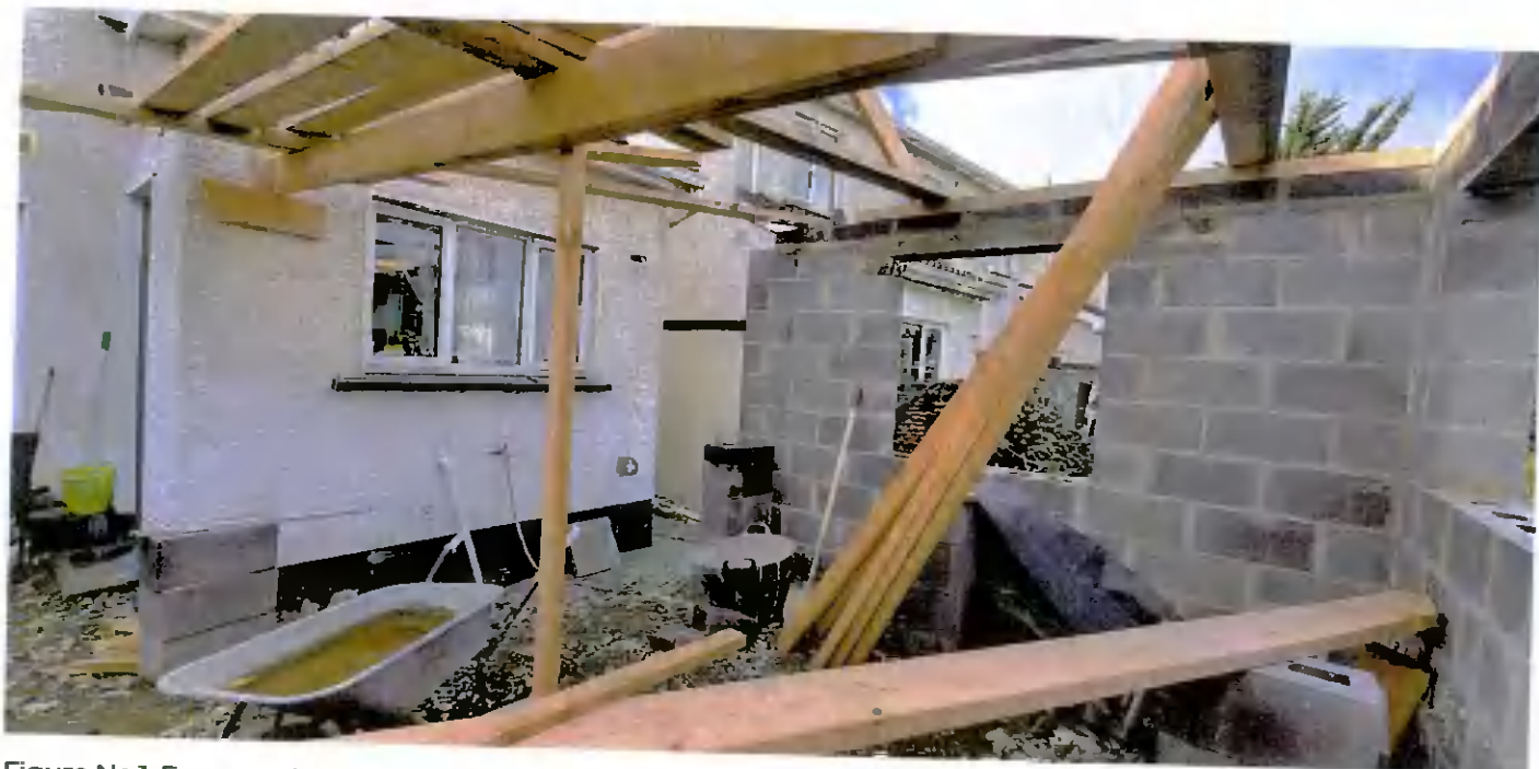
Figure No.1. Exempted Development. Window to the side to be blocked up
