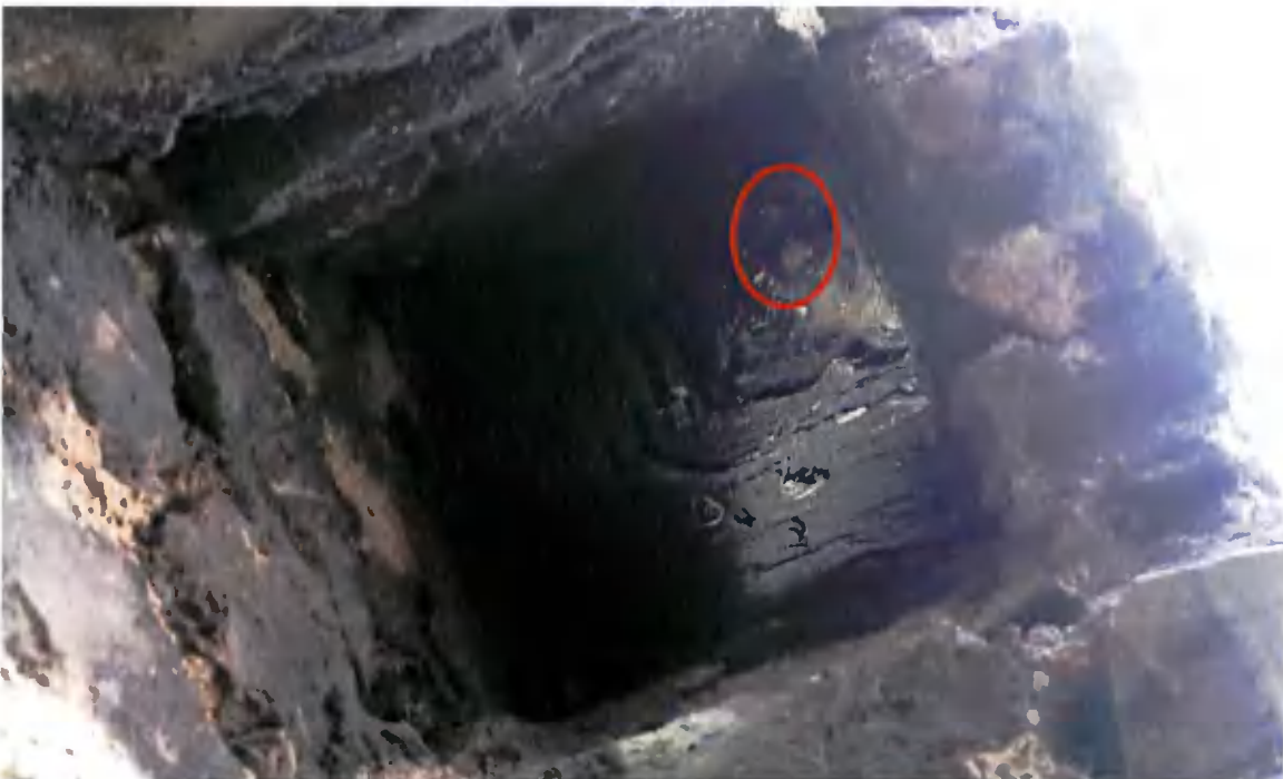
Figure 3-5 Looking up into the chimney, butterfly wings are visible in chimney (red circle)
