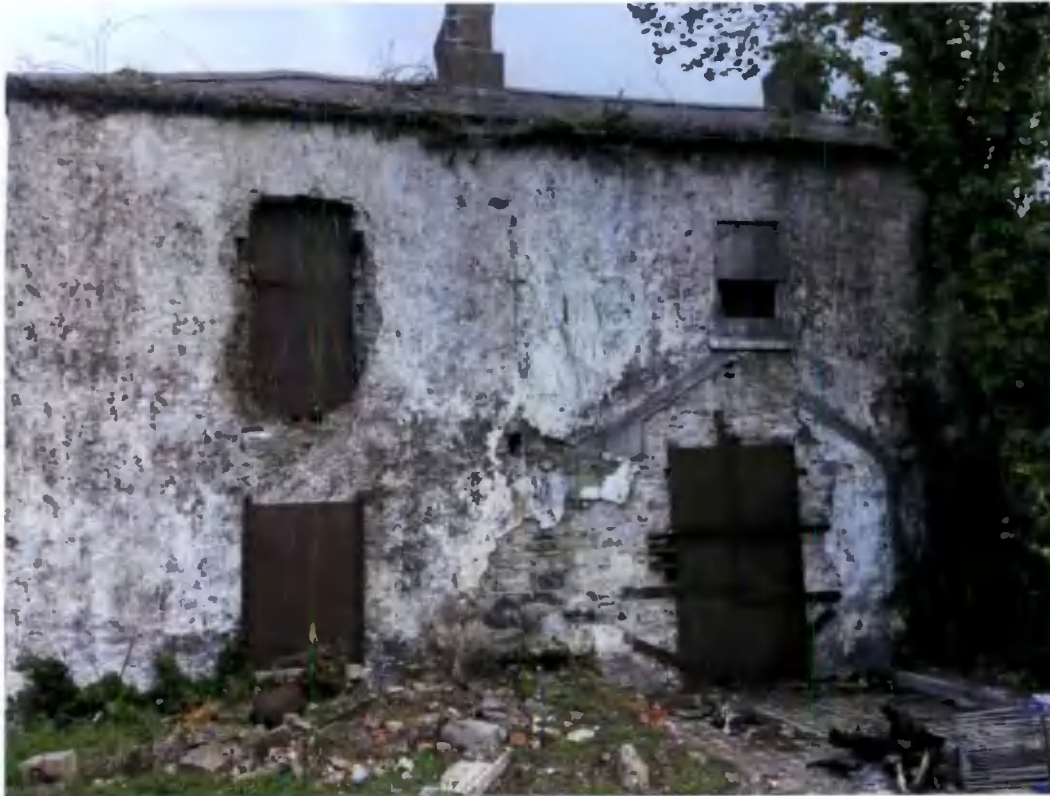
Figure 4-5: Derelict building (Katherine Tynan House).
