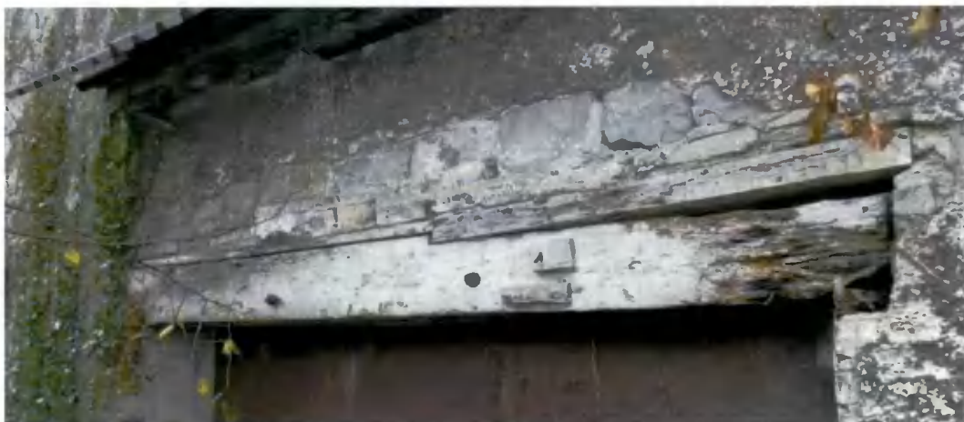
Figure 26: Decay of lintel over large window opening on south elevation
