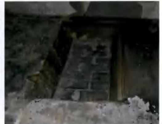
Figure 34: Timber lining to window in room 102
