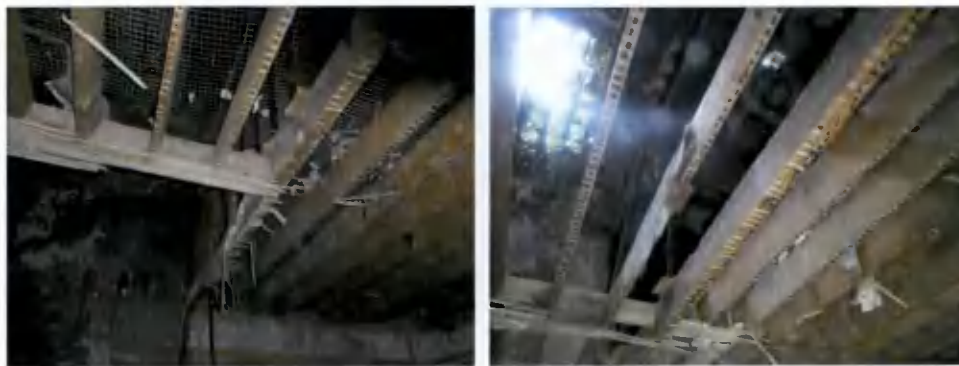
Figure 30: Stairs opening in first floor joists above Room G04 and above Room G01
