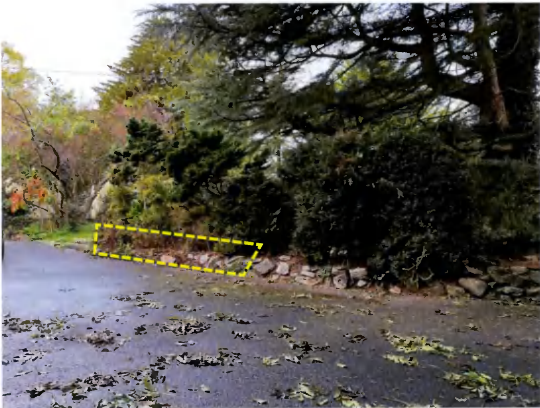
Photo 4: View showing the area within the RPA of the mature cedar (T734) that is required to be reduced in order to construct the proposed driveway and tie in with the existing driveway.
