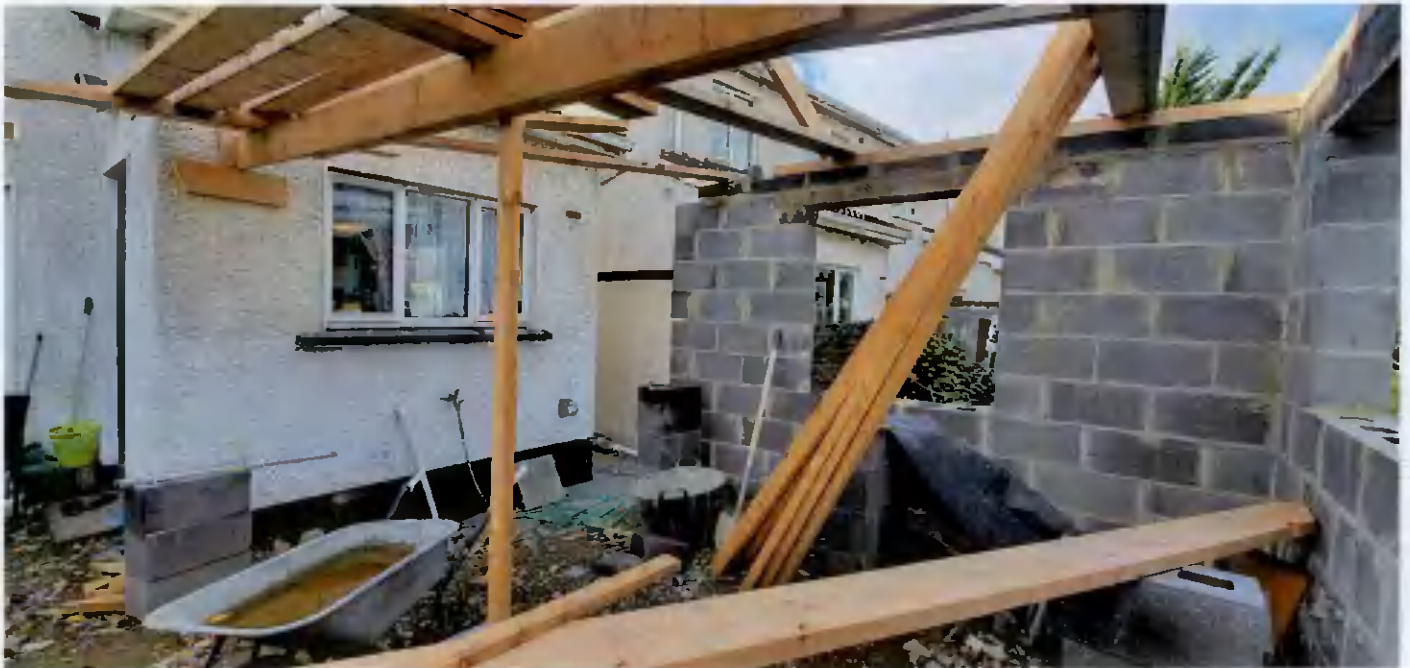
Figure No.1. Exempted Development. Window to the side to be blocked up
